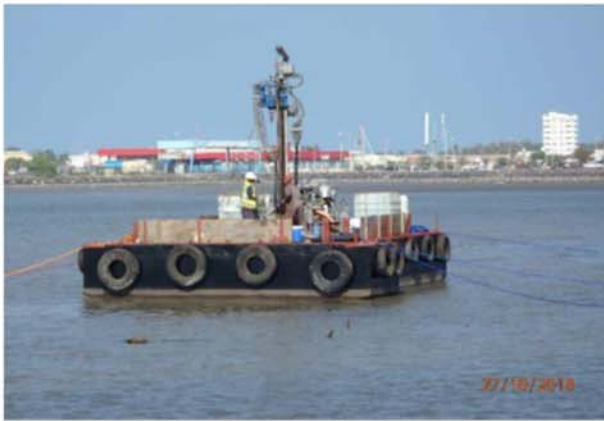
Geotechnical Investigation at Djibouti Port Natural condition survey: Geotechnical investigation by pontoon (Djibouti Port and Tadjourah Port)
