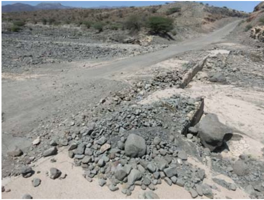
Photo: Damaged Road
