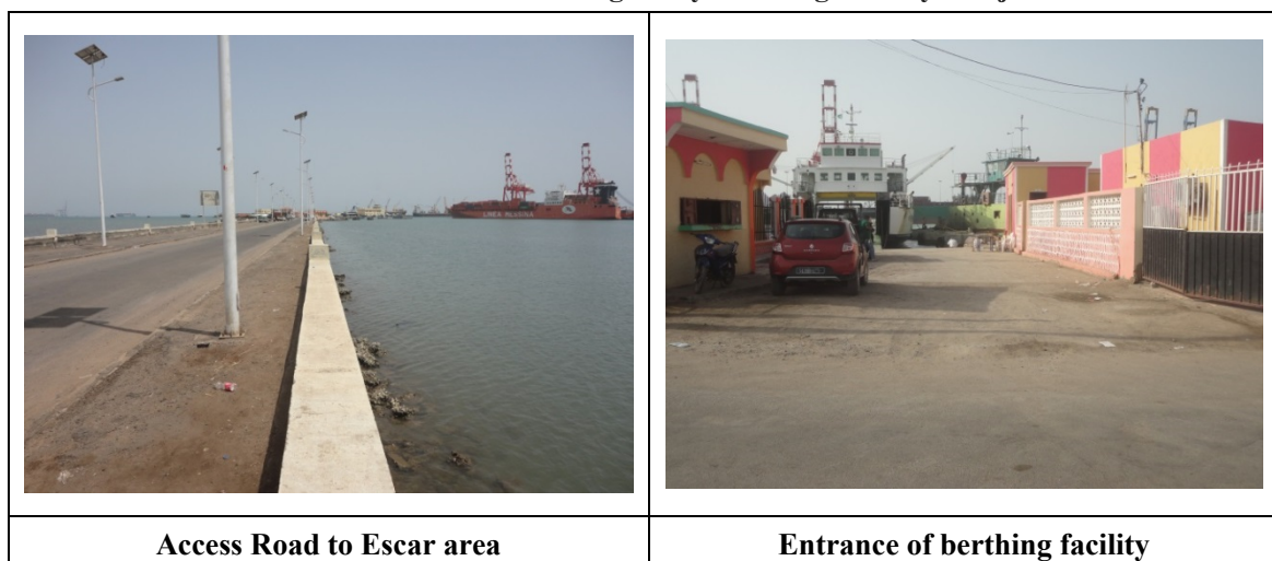
Photo: Current Status of the Existing Ferry Berthing Facility at Djibouti Port
