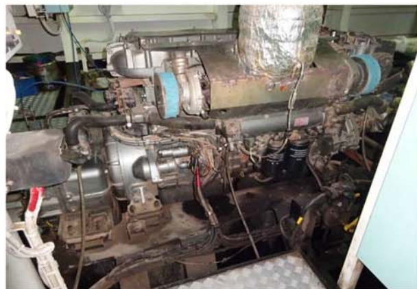
Main Engine for Present Ferry Under poor maintenance (2 nd July 2018)
