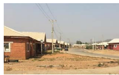
Catenary in the satellite town (final)
