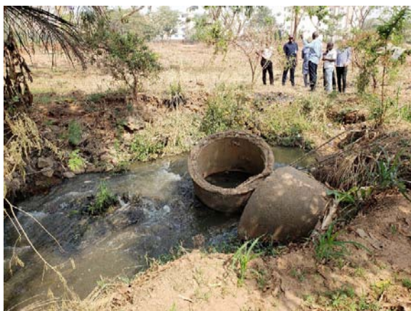
No.3 Damaged Manhole
