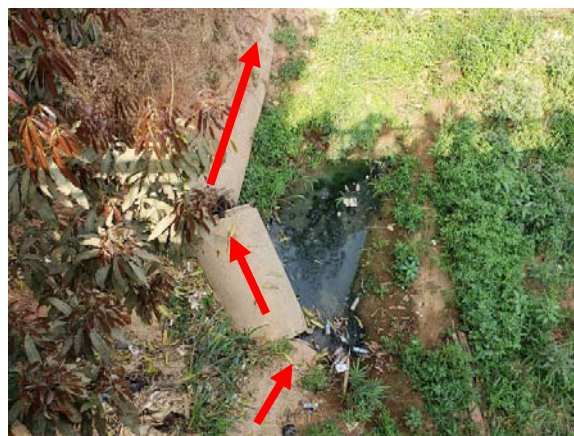
No.4 Flushed Sewer Pipes by Erosion in River Bed
