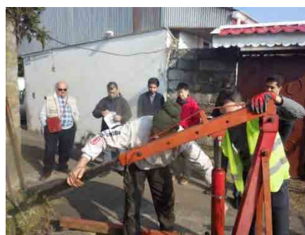
Final inspection of the installation of vacuum chamber with the mission from JICA Iran Office
