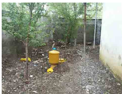
Installed on-site sewage treatment package with RWWC's budget
