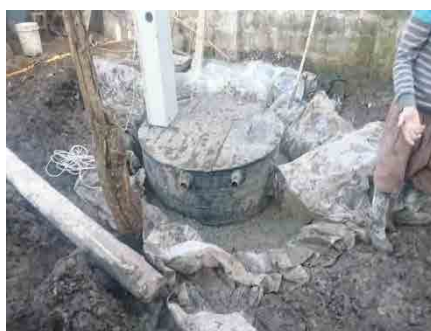
Installed on-site sewage treatment package with JICA's budget to be operated on trial
