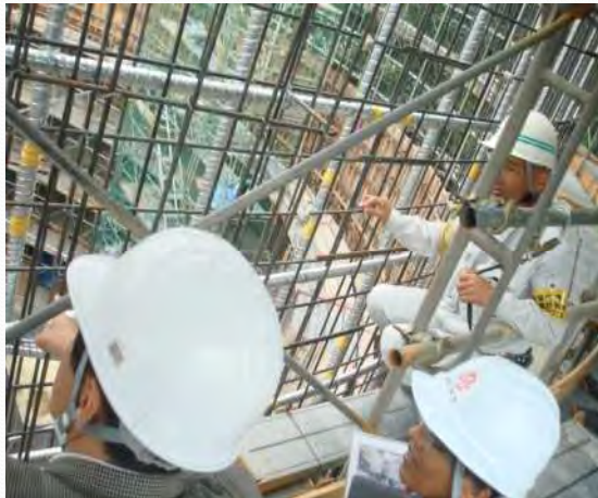
Close up; Form Work+ (Vertical Pre stressing bars+ Horizontal Pre-stressing wires)Inside Sheaths
