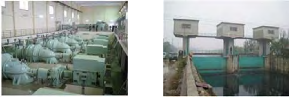
Photo 4.11 The flood countermeasure facilities developed at JICA's "Hanoi Water Environment Improvement Project II" (Left: Yen So pumping station, Right: Tanriet flood control flood gate)
