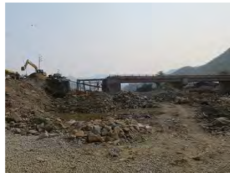
Photo 2.4 A bridge partially lost by flash flood (Son La Province)
