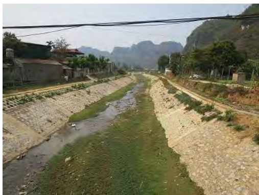
Photo 4.2 Construction of flow pass (Son La Province) Damaged by debris flow, flow path work was done in urban area.
