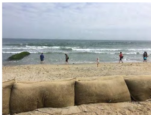
Installation of sandbags (The sandbags are installed parallel to the shoreline as the jetty for accretion of sand)
