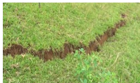
Crack on dike slope Ta Chu River (Thanh Hoa province)
