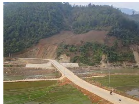
Photo 2.6 The situation of the unstable slope in contact with newly constructed roads and bridges (Yen Bai Province)
