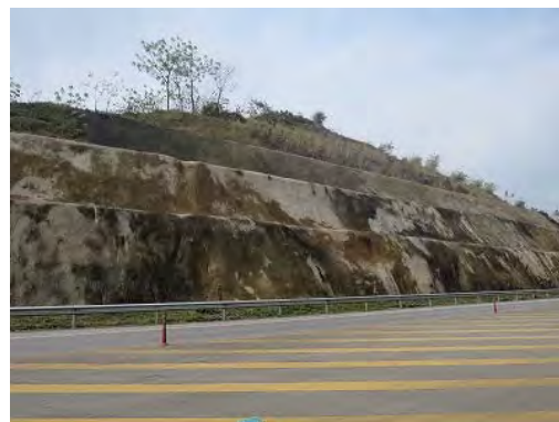
Photo 4.3 Road protection measures along the national road (Lao Cai Province) Cutting, concrete spray, drainage hole has been constructed.
