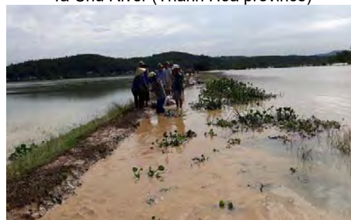
Overtopping into land side and emergency measures (piling sand bags) Huu Hoat river (Thanh Hoa province)
