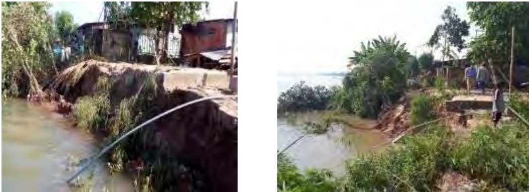
Photo 2.9 View of riverbank erosion damage in Dong Thap Province
