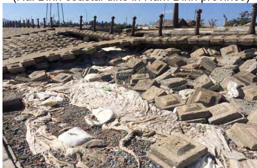
Collapsed revetment on coastal dike (Ha Tinh province)
