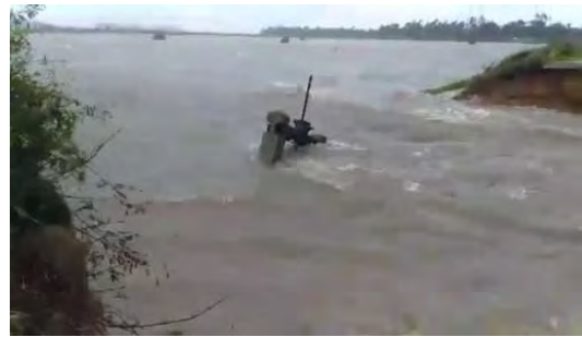
Broken coastal dike and drainage sluice (Ta Nghen dike in Ha Tinh province)
