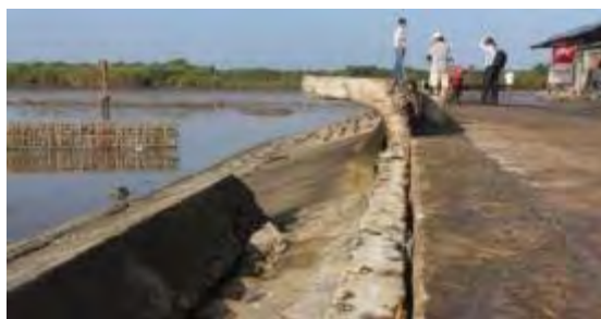
Photo 2.13 View of coastal erosion damage in Bac Lieu Province
