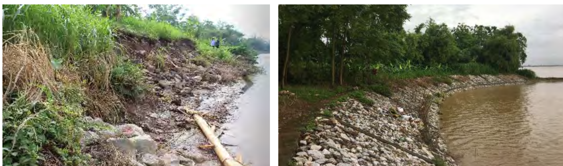
Photo 4.4 View of riverbank erosion in Hung Yen City (Left: before countermeasure, Right: after countermeasure)
