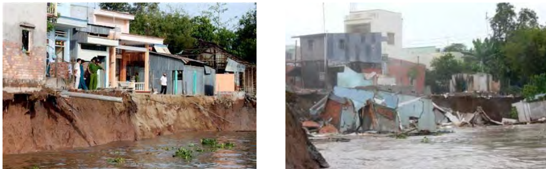
Photo 2.10 View of riverbank erosion damage in An Giang Province
