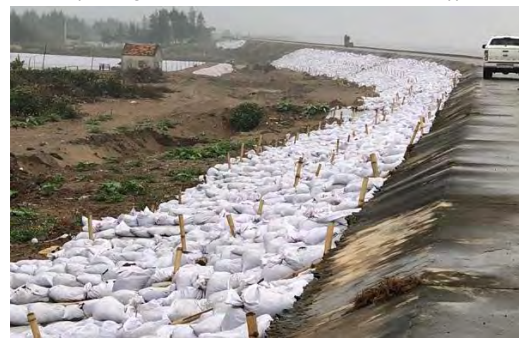
Emergency measures by sand bags to prevent scouring at toe of slope (Nam Dinh province)
