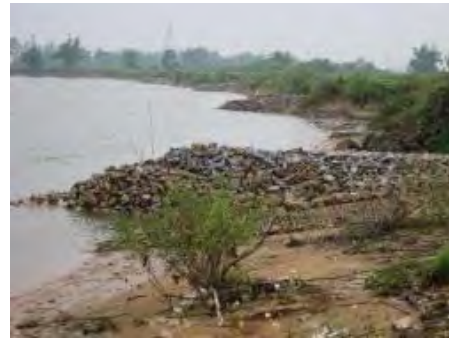
View of repair of a riverbank slope on the La River in Ha Tinh Province (work in progress, April 2015)
