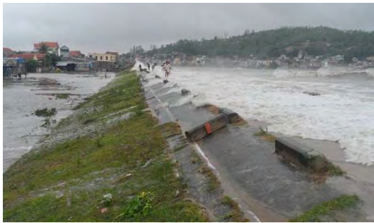
Overtopping due to high tide (Hai Binh coastal dike in Nam Dinh province)
