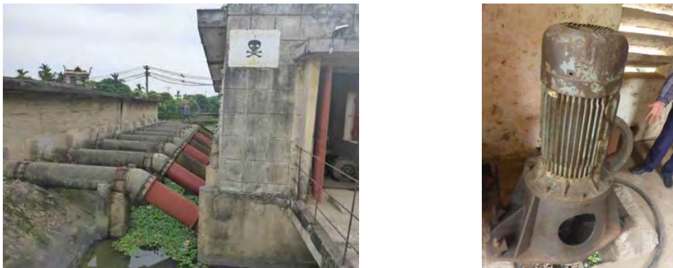
Photo 4.12 Drainage pump facility in Hai Duong province
