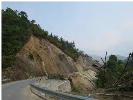
Photo 2.3 Collapse along the prefectural road (Son La Province)
