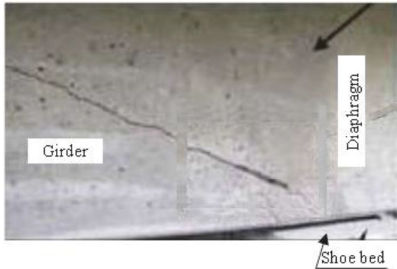
Photo 9-1 Example of Shear Crack
