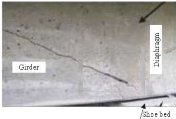
Photo 10-1 Example of Shear Crack
