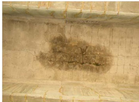
Damaged Deck Slab with water leakage
