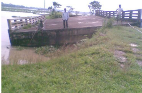
Photo 3-14-1 typical Bridge scour
