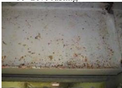
Photo18-1 Surface area of 10~20% rusting
