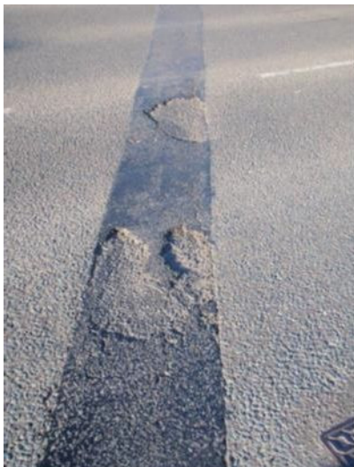
Damaged Asphaltic plug joint
