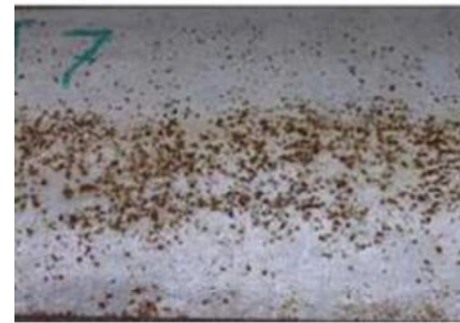
Photo18-2 Surface area of 20~30 rusting
