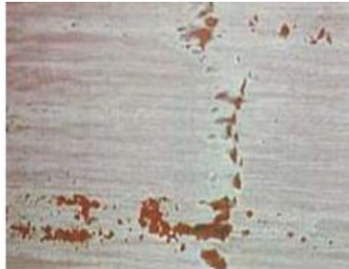
Photo18-3 Less severe corrosion
