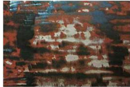
Photo18-4 More severe corrosion
