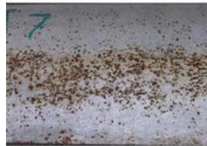
Photo4-2 Surface area of 20~30 rusting
