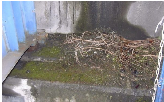
Fig.2-10 Bearing with Debris
