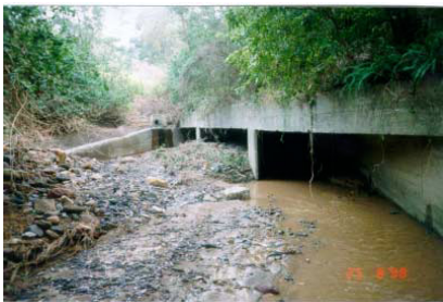
Fig. 2-16 Culvert with flow obstruction
