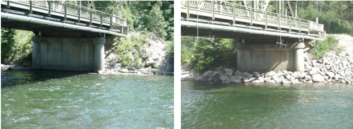
Figure 4-14 Scoured bridge pier (left) and after Repair work (right)
