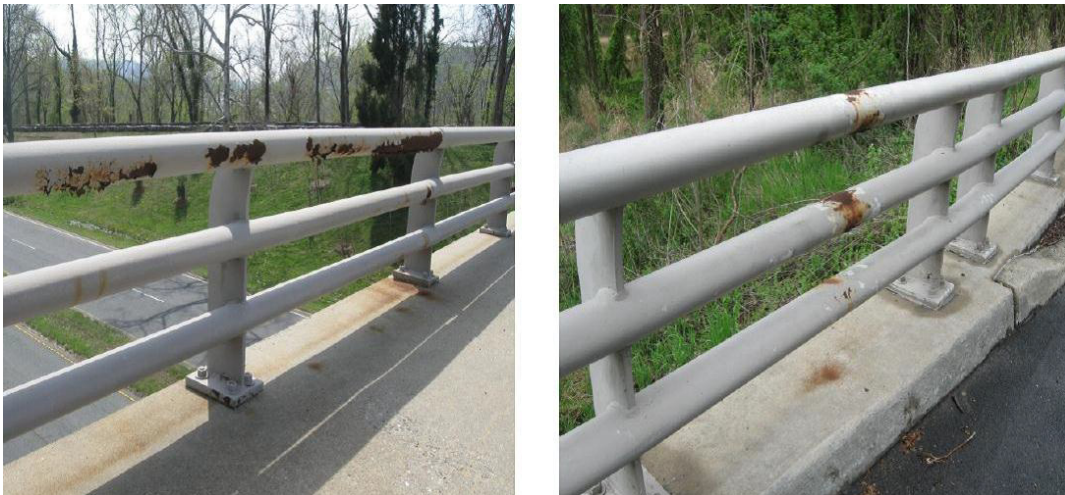
Figure 4-16 Rusted Railings with Flaking Paint that Require Spot Painting
