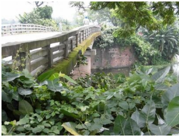
Fig.2-17 Harmful weed around the bridge
