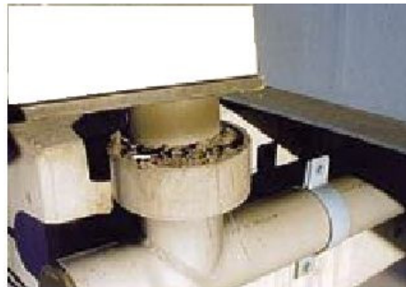
Fig.2-5 Blocked drain pipe with bird's dung
