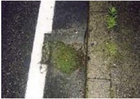
Fig.2-3 Blocked catch basin at surface
