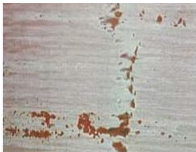
Photo4-3 Less severe corrosion
