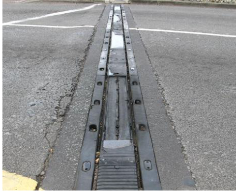
Figure 4-7 damaged Expansion Joint
