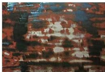
Photo4-4 More severe corrosion
