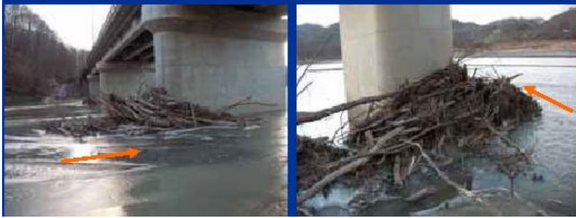
Fig. 2-14 Pier with flow obstruction
