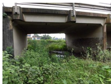
Fig. 2-18 Harmful weed under the bridge
