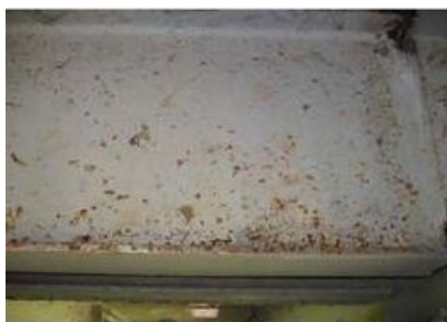
Photo4-1 Surface area of 10~20% rusting
