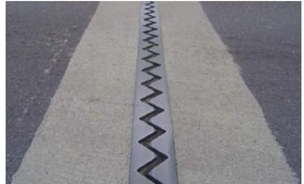
Figure 4-8 Steel Expansion Joint
