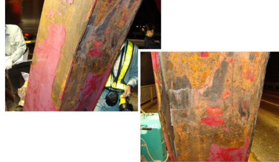
Main girder is deformed and cracked due to traffic collision.
