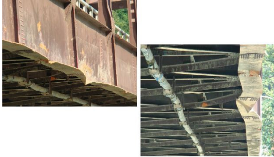
Main girders are deformed and damaged due to flood water.
