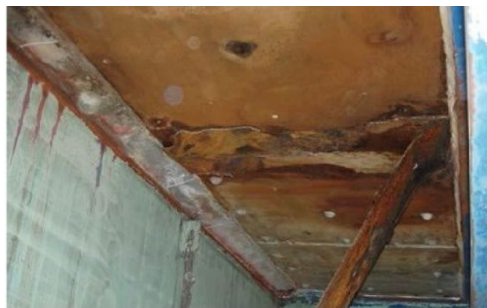
Falling off of the deck slab reinforcement steel
