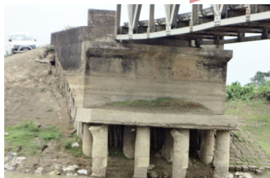
Pile foundation Largely exposure of the footing underside
