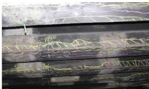
Fire damage of concrete girder
