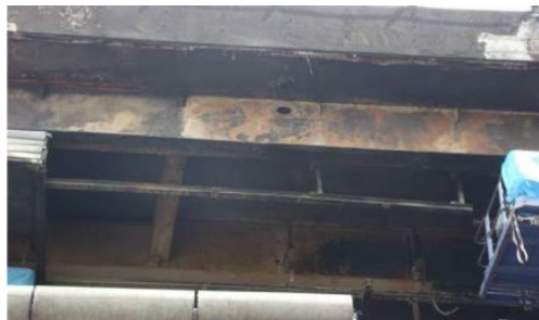
Fire damage of steel girder
