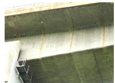
Rust stain at construction joint
