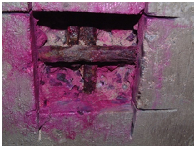
Photo-6.3.7 Phenolphthalein method by exposed rebar and Rebar corrosion
