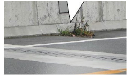
Accumulated debris such as overgrown weeds
