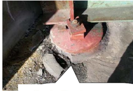
Break of bearing seat mortar
