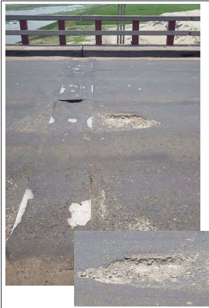
Photo 5: Pothole near expansion joint
