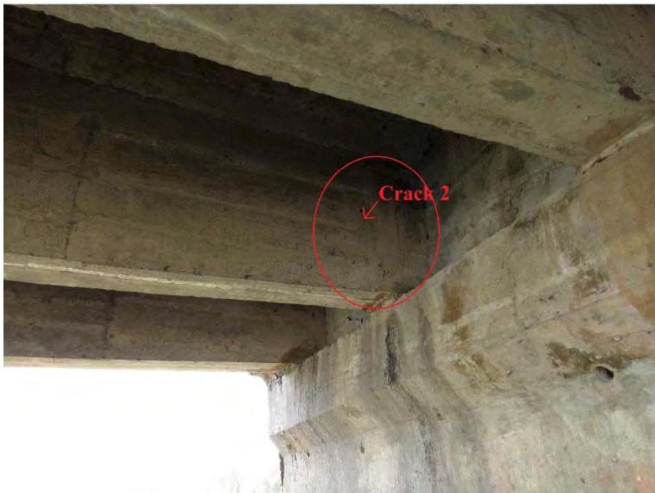
Photo 2-2 Position of Crack-2
