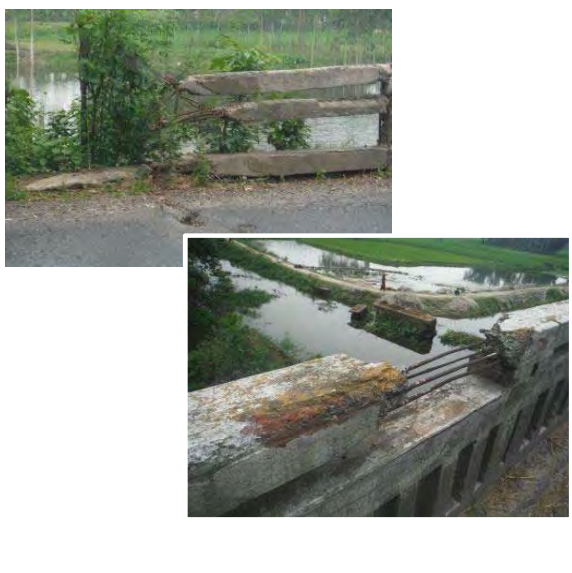
Photo 4 Spalling/Rebar exposure of railing
