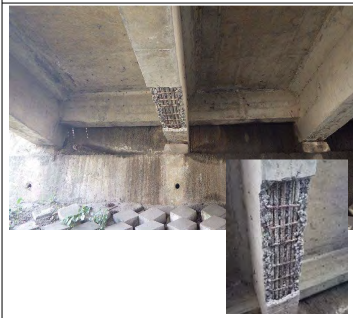
Photo 7: Spalling & Exposed Rebar on Main Girder (A2, Rajshahi End)
