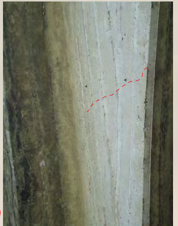
7 G3 : Cracks of Main Girder
