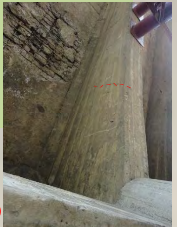
8 G2 : Cracks of Main Girder
