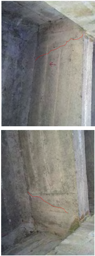
Photo No.3 A1-P1 G3 : Shear Cracks of main Girder
