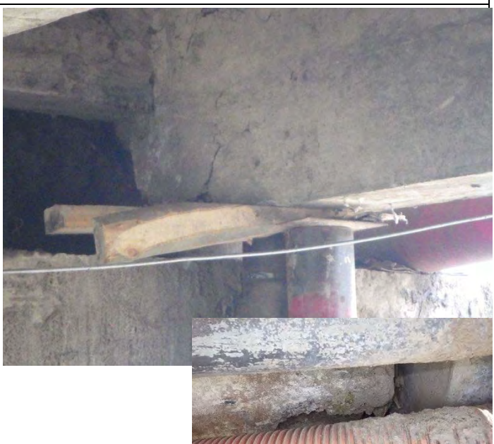
Photo 8: Crack & Spalling on Main Girder (P1, Dhaka end side)
