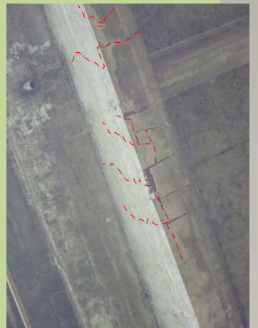
9 G1 : Cracks of Main Girder
