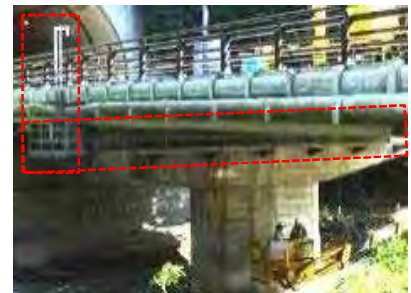
Example: Inspection Platform and Ladder
