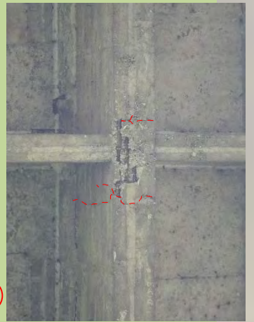
10 G2 : Cracks of Main Girder
