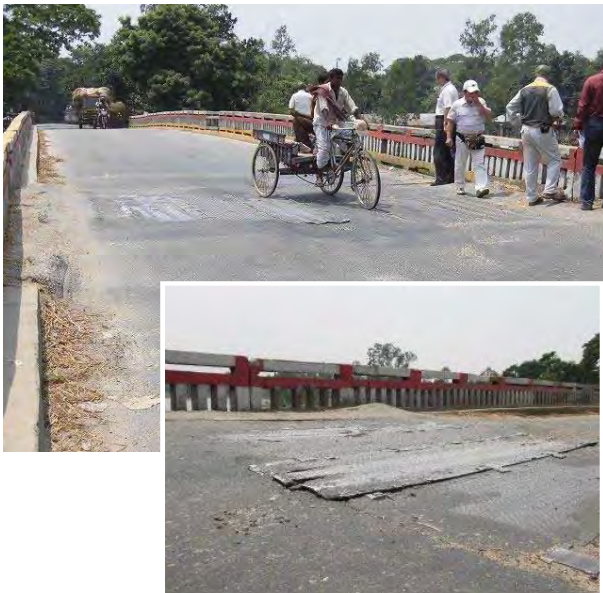
Photo 3 Damaged surface with steel plate as temporary measure
