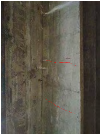
Photo No.5 AI-P1 G1 : Flexural Cracks of main Girder
