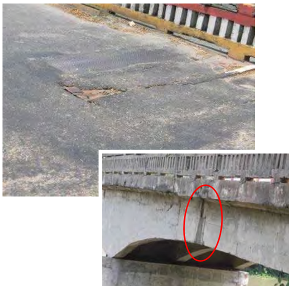
Photo 5 Damaged expansion joint above Gerber-hinge
