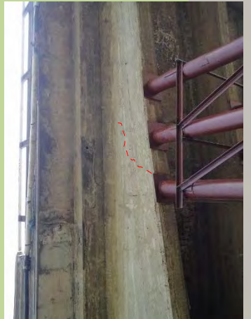
5 G3 : Cracks of Main Girder
