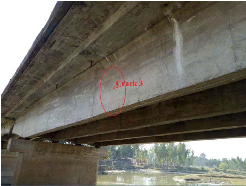
Photo 2-3 Position of Crack-3
