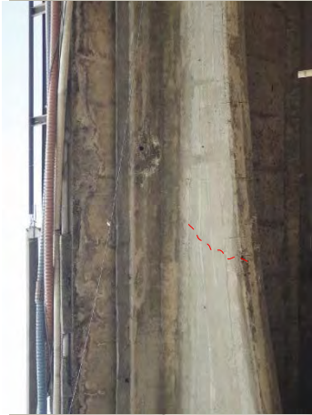
2 G1 : Cracks of Main Girder
