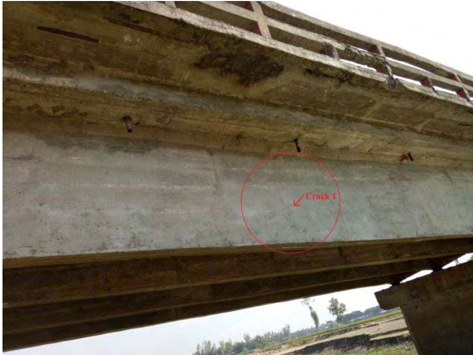
Photo 2-1 Position of Crack-1
