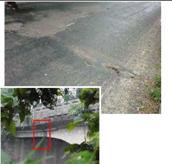
Photo 6 Buried expansion joint above Gerber-hinge
