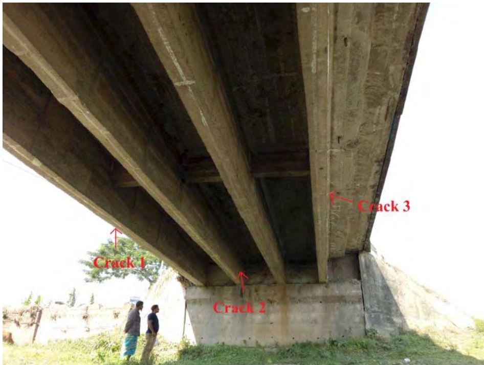
Photo 2-4 Position of Crack-1 to Crack-3
