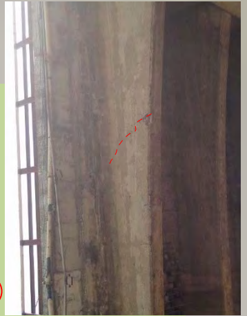
6 G3 : Cracks of Main Girder
