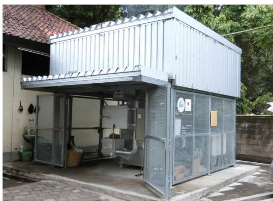
Compact incinerator installation (Wangaya Hospital)
