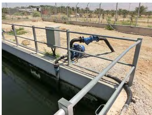
Photo-3 Irrigation Pump
