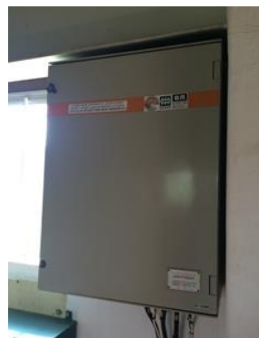
Existing Remote Technical Unit
