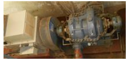
Chilanga Booster Pumping Station
