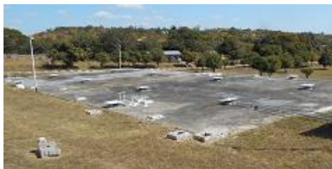
Treated water reservoir in Iolanda Water Treatment Plant
