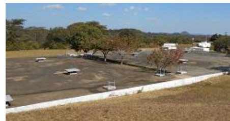
Treated water reservoir in Chilanga Booster Pumping
