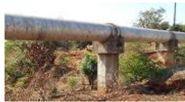
Water transmission steel pipe φ 900 mm
