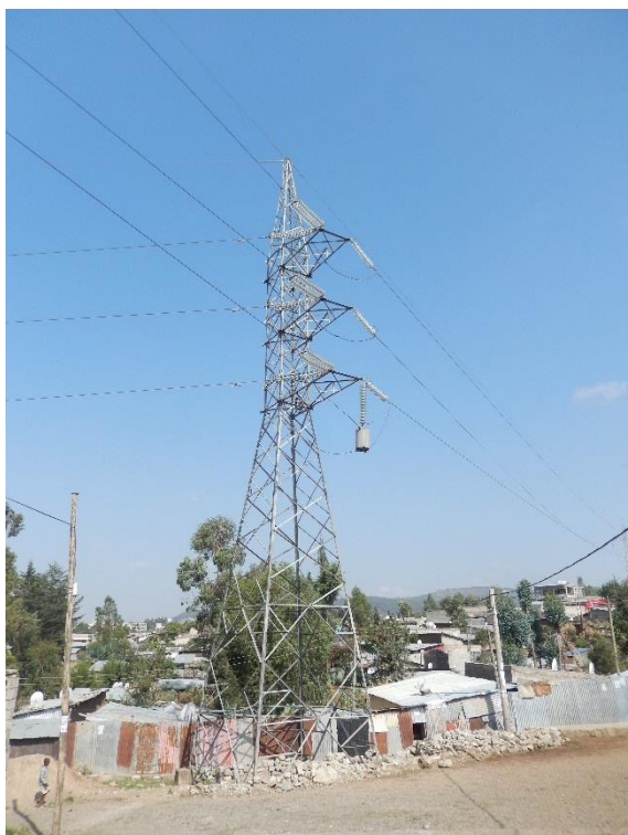
T 62 DSCN0444 T-Branch to Weregenu Substation
