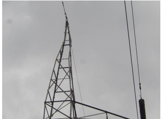
T38 DSCN0743 T38 Ground Wire arm was damaged and bend. Arm can be callapes in any time.
