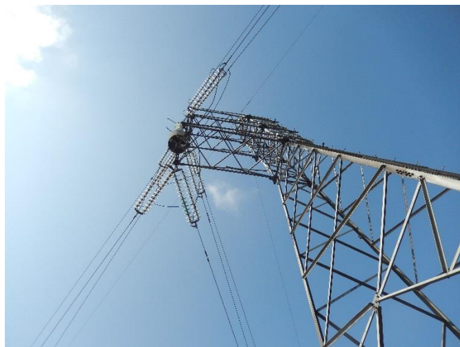
T 62 DSCN0454 Kaliti-I to Cotebie Transmission Line
