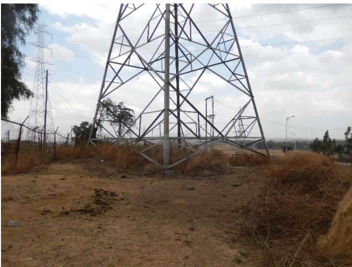
DSCN0867 T55 bottom T55 has many missing steel members.
