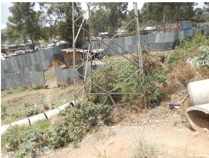
T 34 DSCN0485 T34 beside road. Water drain pipes for road are installed beside tower foundation.
