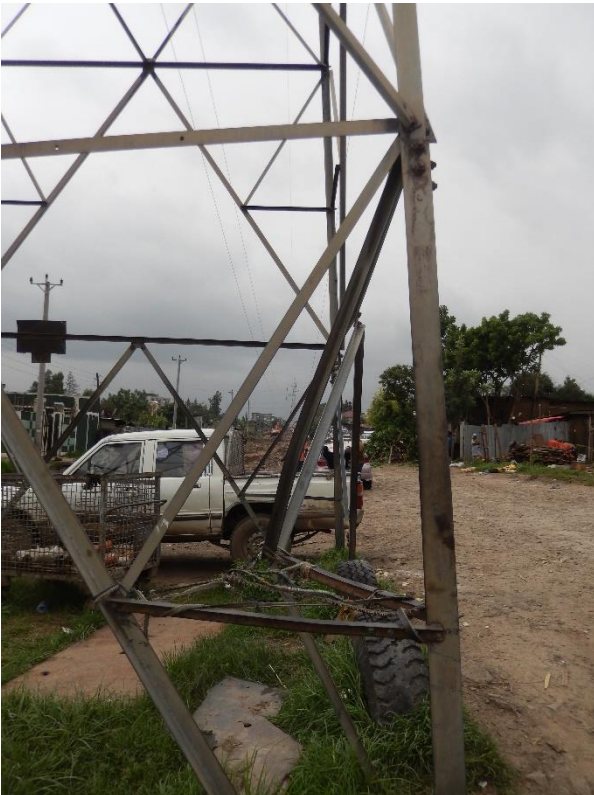
T18 Damaged Leg steels
