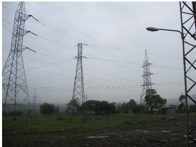
T 56 IMG_1244 down lead to gantry from T56 & T55
