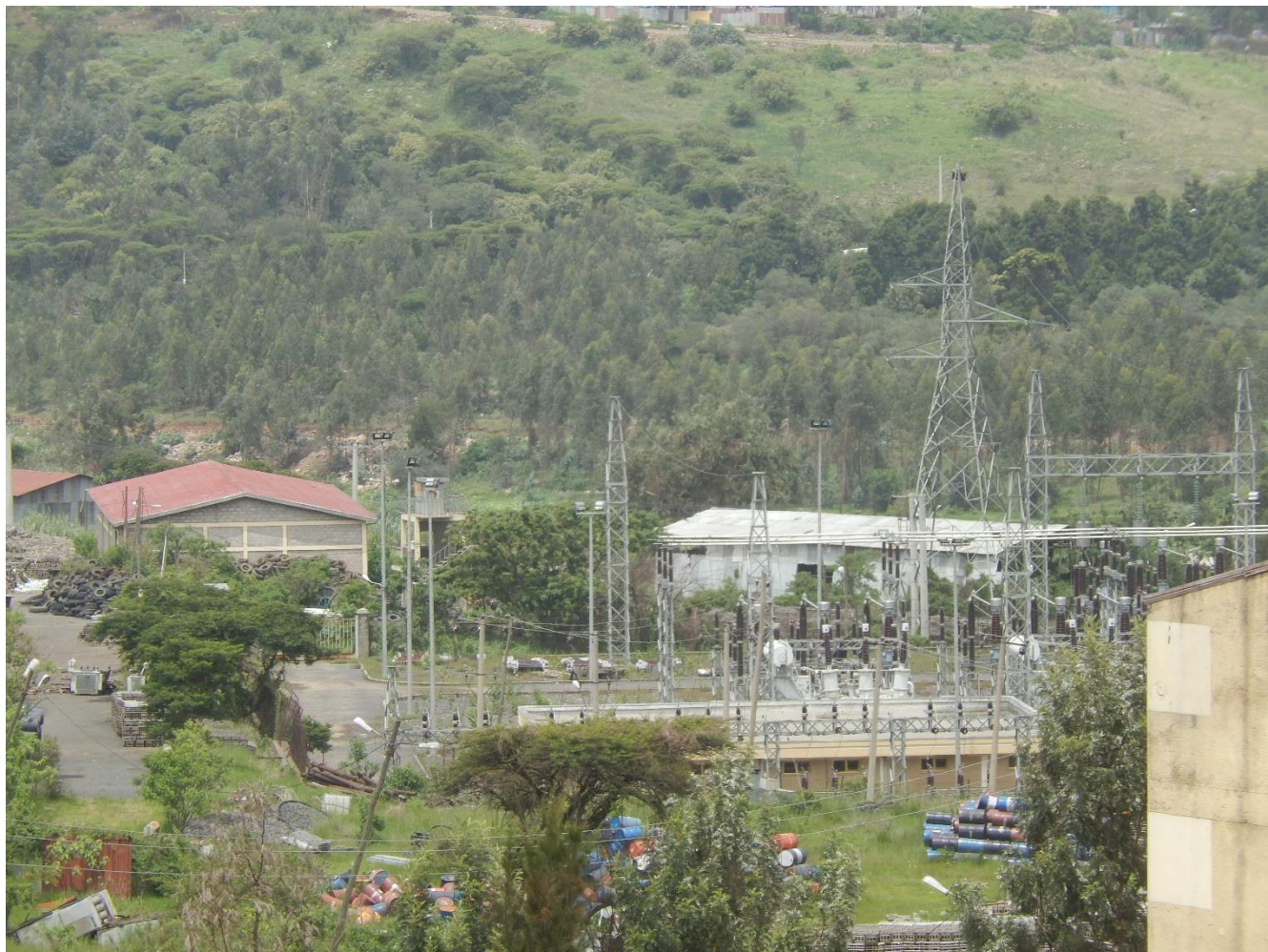
Gofa Substation (Addis South II) P1130584 Gofa SS from T20 (photo 20 th 2018 June)
