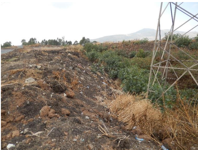
T 41 DSCN0775 T41 foundation level is much lower than existing ground level of water treatment facility.
