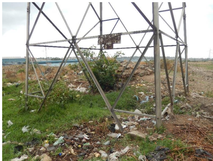
T35 Ground elevation level become higher than original ground due to embankment by construction of new industrial factory area.
