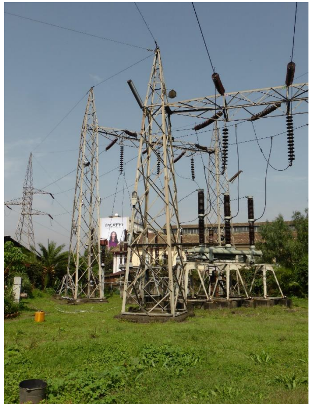
Addis Center Substation at 7 th July 2017. A Plan for Substation modification is considered.
