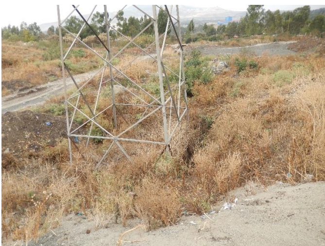
T 42 DSCN0784 T42 bottom T42 foundation level is much lower than exiting ground level of water treatment facility.
