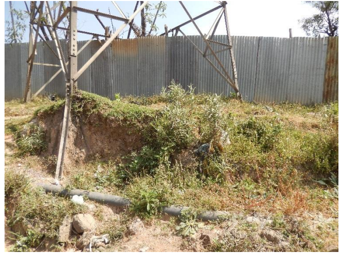
T52 Kaliti – Sebeta Existing Foundation Two steel angles were used for each leg to support tower
