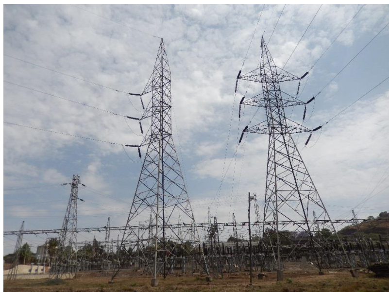
DSCN0960 T56 to gantry of Kaliti-I substation.
