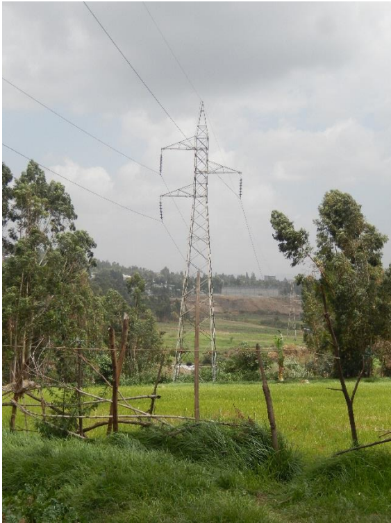
T 39 DSCN0768 T39 from T40. T 39 – 40 -41 is transposition tower.
