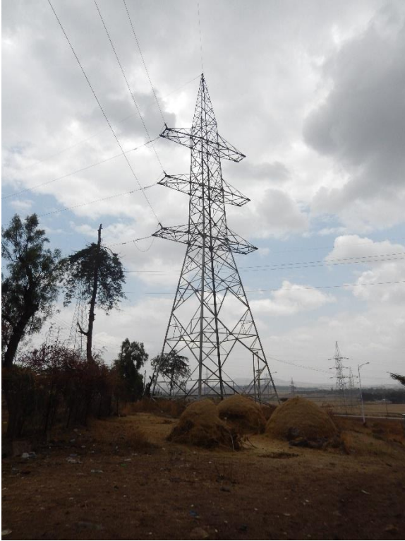
T 55 DSCN0866 T55 from T54 220kV Dead and tower.
