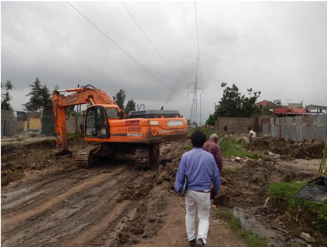
Obstruction houses on right side has been removed now. Tower 17 is damaged by construction and slightly declined.
