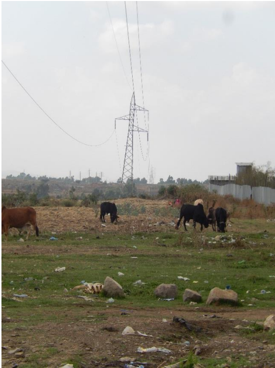
T 36 viewed from T35. DSCN0707 T36. Tower is in inclineing.
