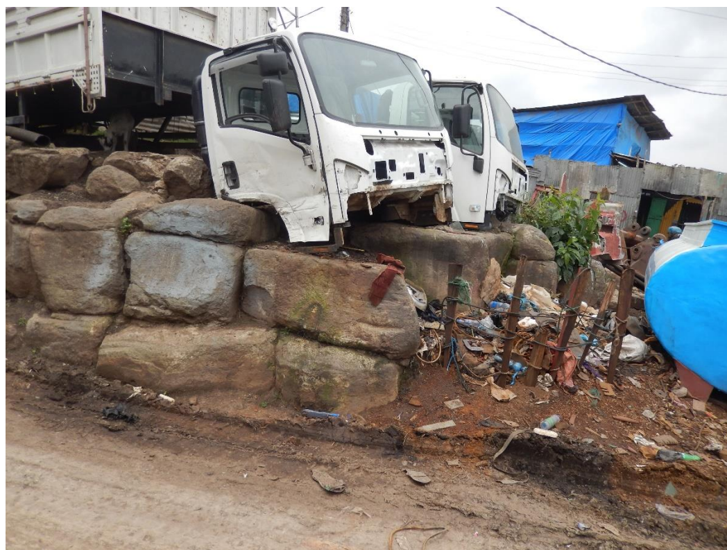
T20 on the slope toward existing road. Here will be end of new construction road
