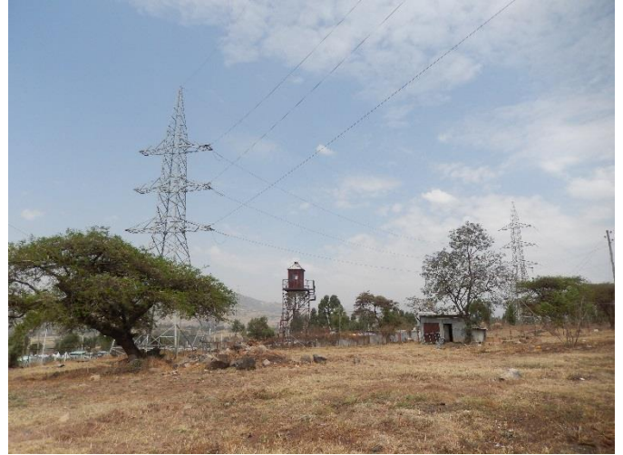
T 55 DSCN0953 T55 from inside Kaliti-I substation.
