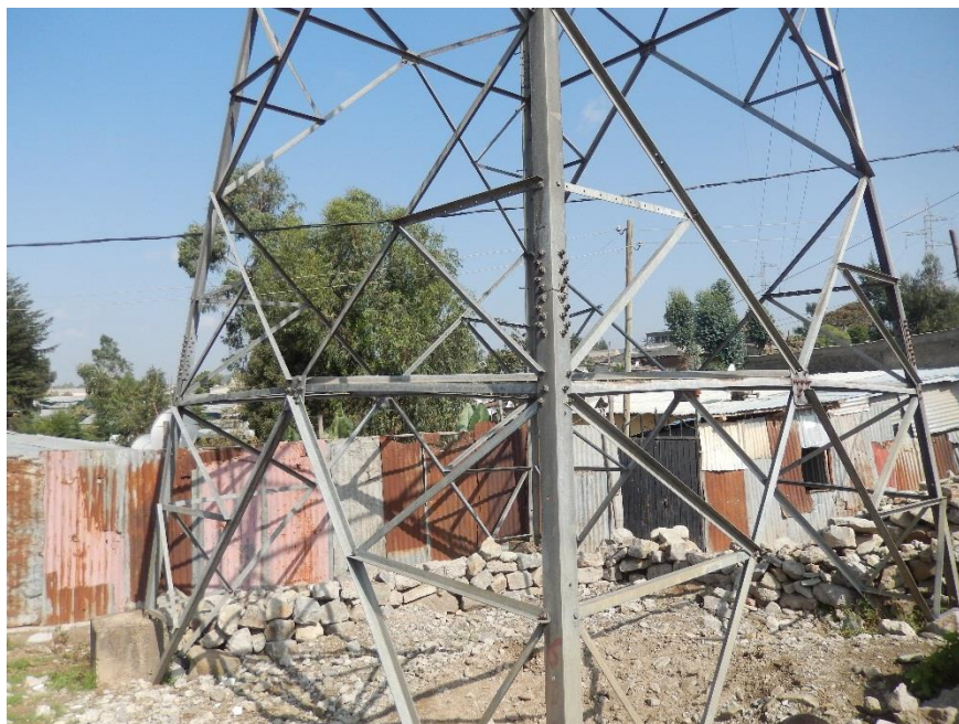
DSCN0452 First horizontal members are all bent
