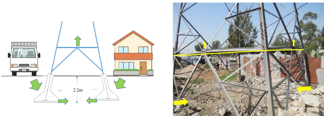
Fig. 7.1-6 Deformation by Soil Pressure of road and houses
