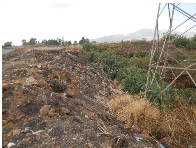
T 41 DSCN0775 T41 foundation level is much lower than existing ground level of water treatment facility.
