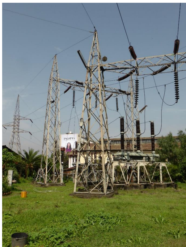
Addis Center Substation at 7 th July 2017. A Plan for Substation modification is considered.
