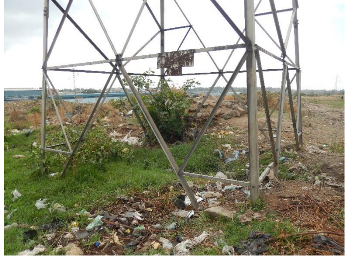
T35 Ground elevation level become higher than original ground due to embankment by construction of new industrial factory area.
