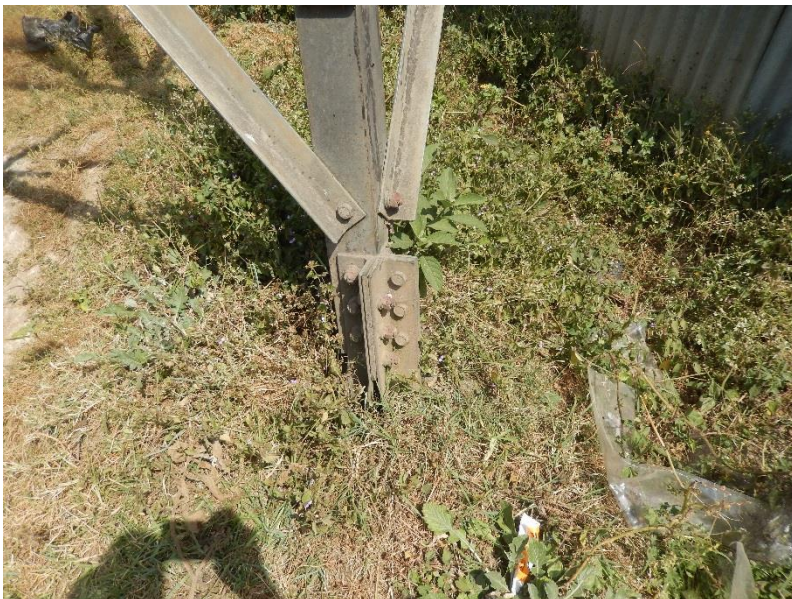
T52 Kaliti – Sebeta Details of connection between stub and tower main leg.
