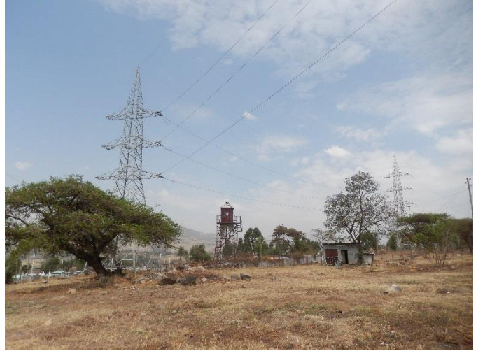
T 55 DSCN0953 T55 from inside Kaliti-I substation.
