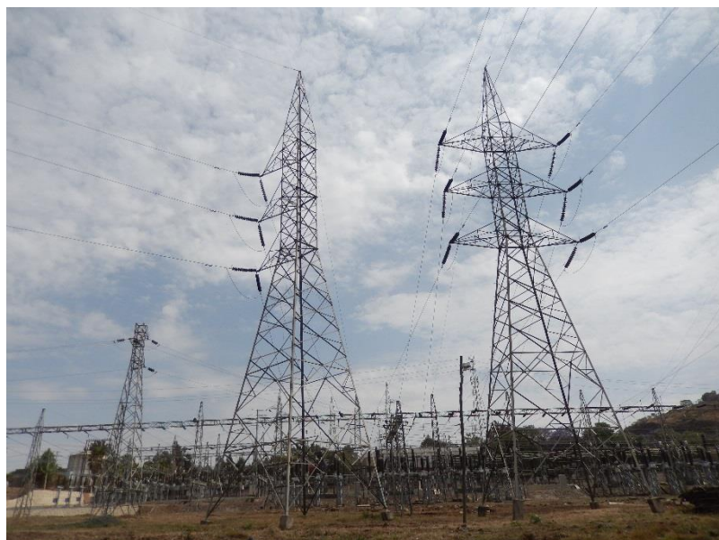
DSCN0960 T56 to gantry of Kaliti-I substation.
