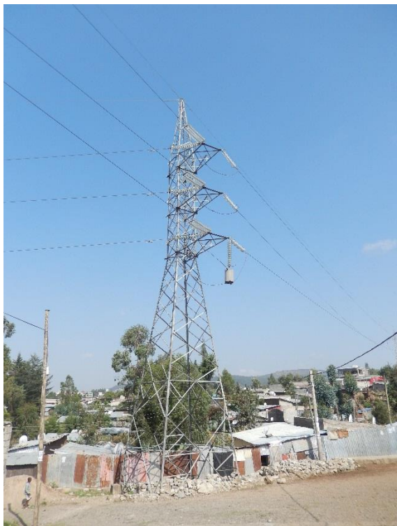
T 62 DSCN0444 T-Branch to Weregenu Substation
