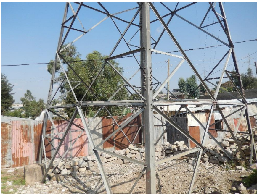
DSCN0452 First horizontal members are all bent
