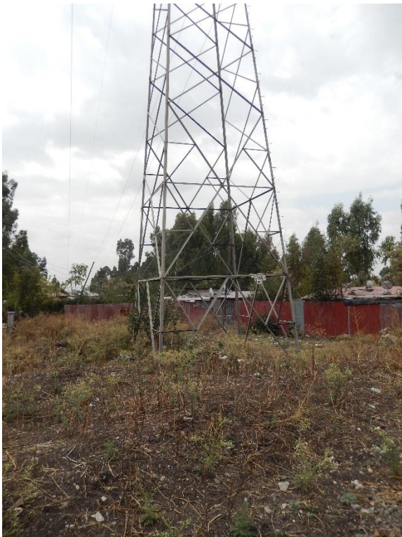
T 43 DSCN0792 T43 beside houses.
