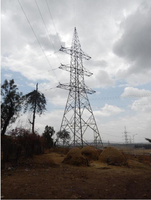
T 55 DSCN0866 T55 from T54 220kV Dead end tower.
