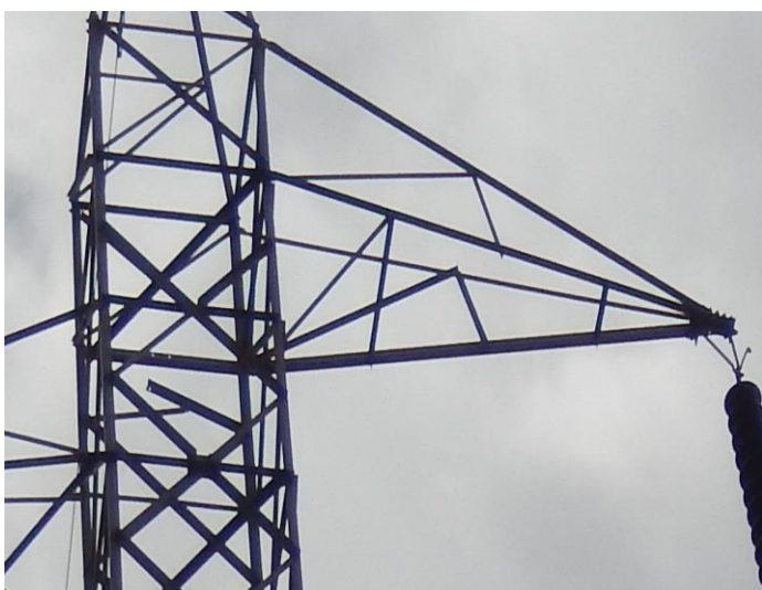
T 45 DSCN0802 T45 top plate are missing or not installed.
