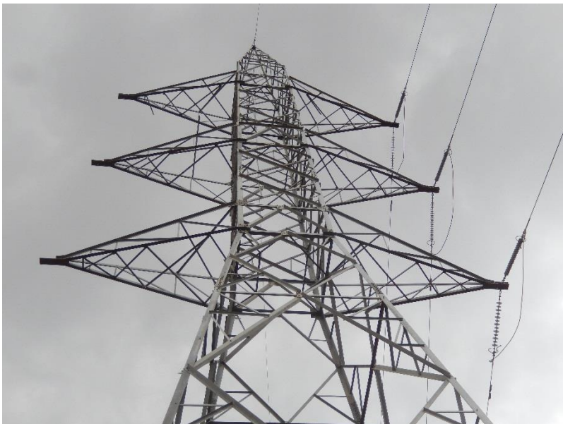
DSCN0865 T54 has many missing steel members.
