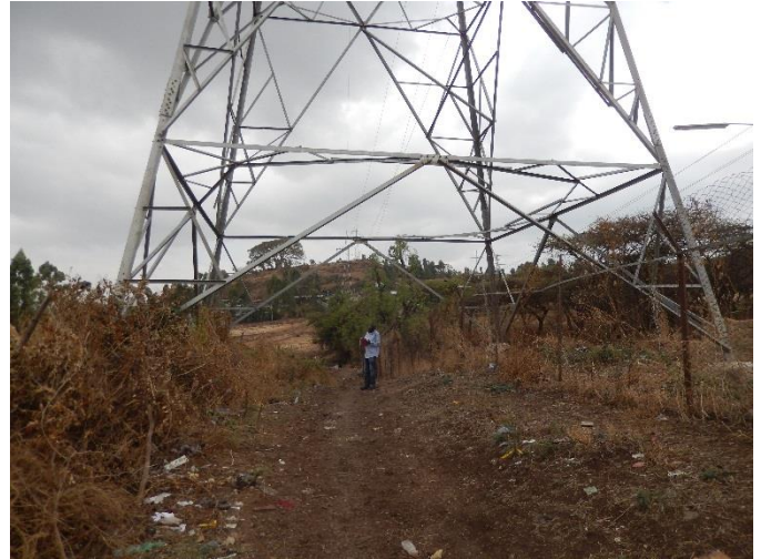
T 54 DSCN0863 T54 bottom Two legs are located out side the Kaliti-I Substation.
