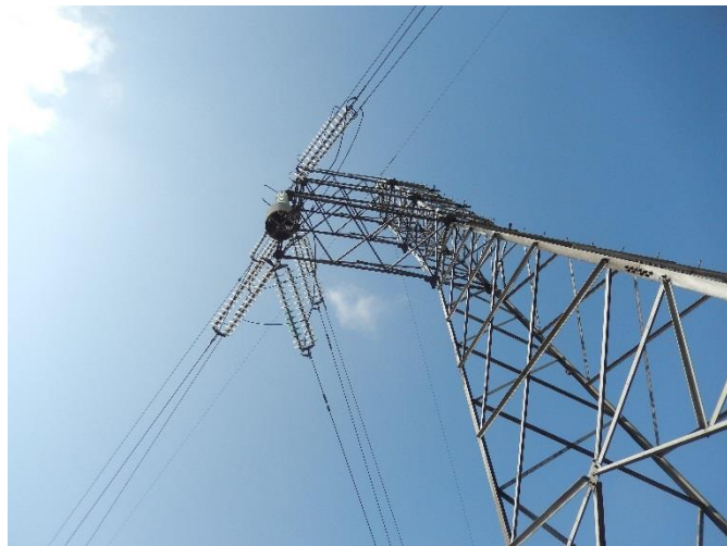
T 62 DSCN0454 Kaliti-I to Cotebie Transmission Line
