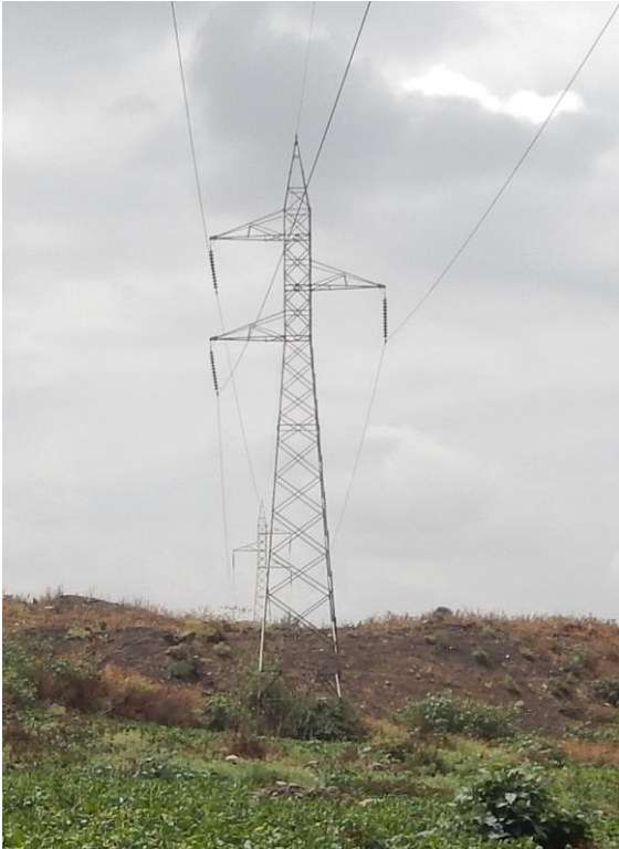
T 40 DSCN0772 T40 from T39 side. The Conductor is inclined due to transposition.
