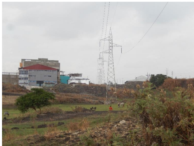
T48 DSCN0826 T48 from 49 Plates for tower cross arm are missing
