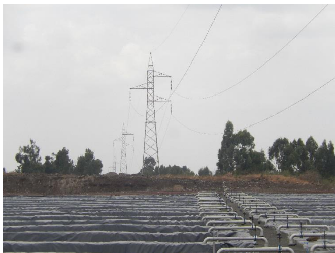
T42 DSCN0778 T42 from T41 Transmission line pass the area of water treatment. An access road is belonging to water treatment. ROW (Corridor) is not so clear, but no houses.
