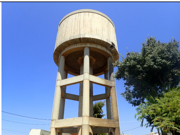
A reservoir with a capacity of 500 m 3 in Sibline municipality, which is to be repaired. Its leakage is estimated at 40 m 3 / 7 hrs, according to inspection by the municipality.
