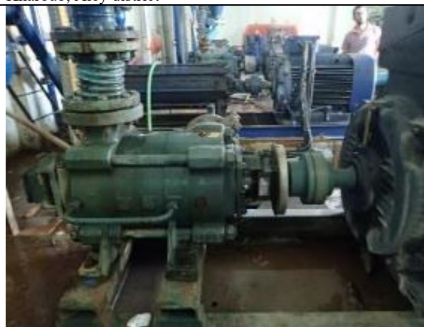
Five water pumps in Jbeil Byblos, occasionally suffering from troubles due to its deterioration. The replacement of three water pumps were requested.
