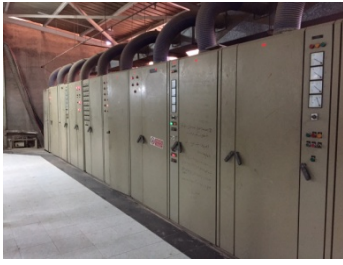
Electrical Panel (Testing at the first location)
