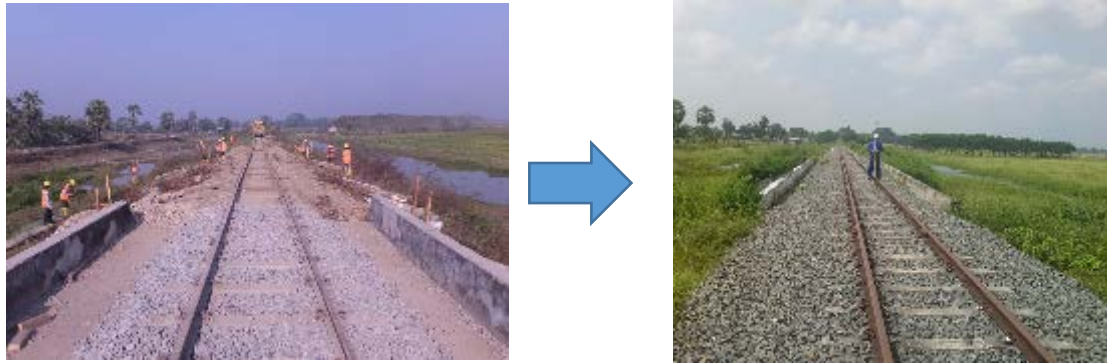
Image-4 Subsidence at the Railway Track Caused by the Subsidence of Ballast (Subsidence volume was approximately 1 ~ 3 cm as a result of the one year observation)
