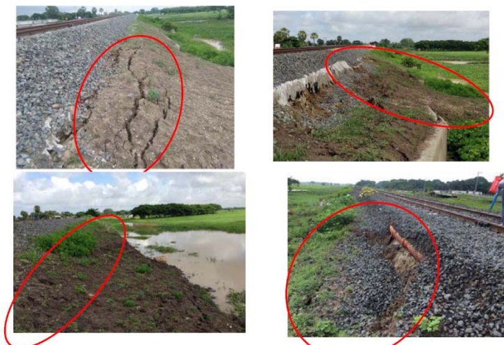
Figure 4.6-2 Situation of slope collapse in the construction in Aizawa (Sliding occurs even in 1:3 inclination)
