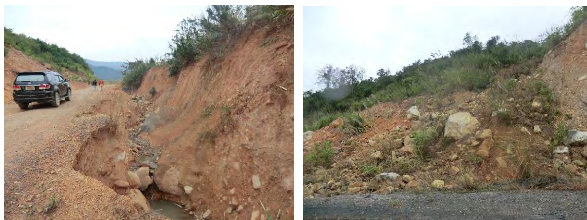
Figure 5.4.6 Conspicuous Slope Failure along Existing Road in the Mountainous Area (at 245 km point of Pre F/S route)
