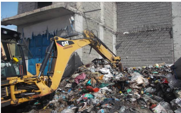
Image 3-14 Removal of market waste (1)
