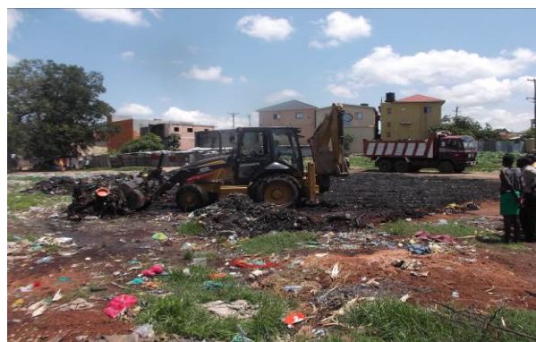
Image 3-17 Illegal dumping behind market
