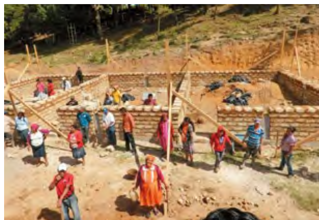
A project to construct a school building using local resources. Each of the 13 community groups works every day in turns. Staff members from the city association in Honduras provide advice so that Ministry of Education standards are met. (Honduras: Project for Strengthening of the Capacity Development of the Local Governments for Regional Development)
