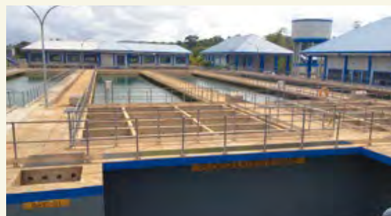
Kandana Water Treatment Plant in Kalutara District, expanded through ODA Loans
