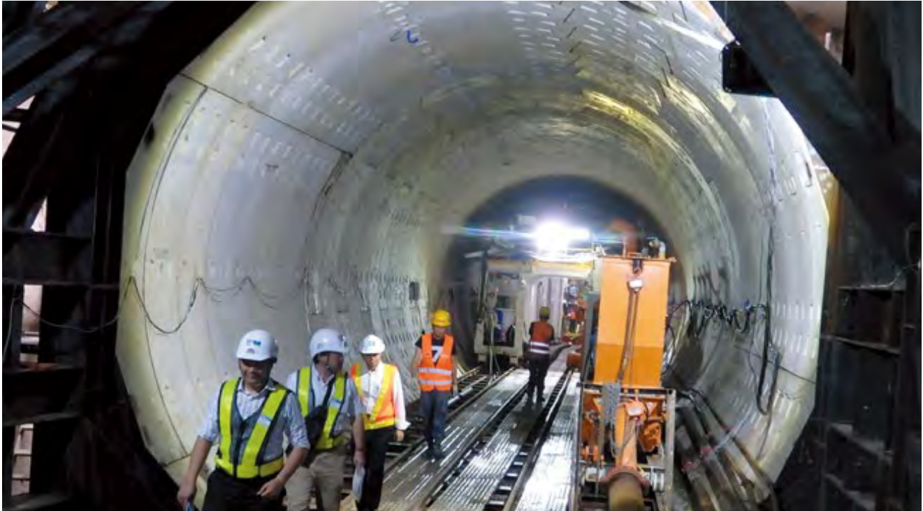
Viet Nam: A construction site of the Ho Chi Minh City Urban Railway Line 1, between Opera House and Ba Son stations. An underground tunnel is being constructed with the shield tunneling method.
