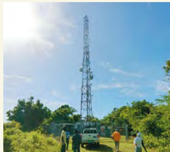
A pylon on which a digital radio antenna will be mounted. A total of 24 such pylons will be constructed throughout the country.
