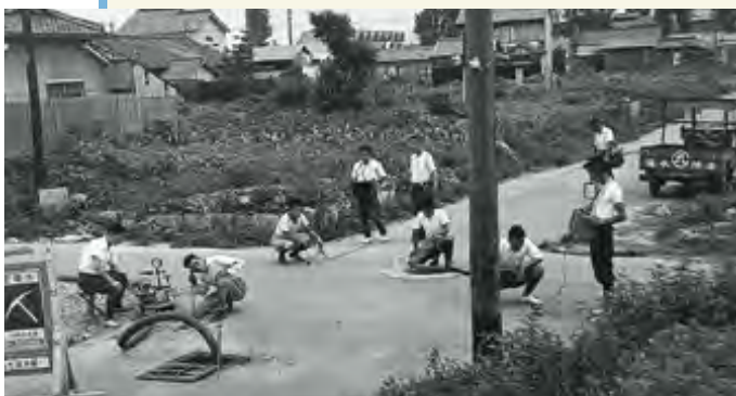
A water leakage check by Nagoya City Waterworks and Sewerage Bureau in the aftermath of World War II, circa 1949.
