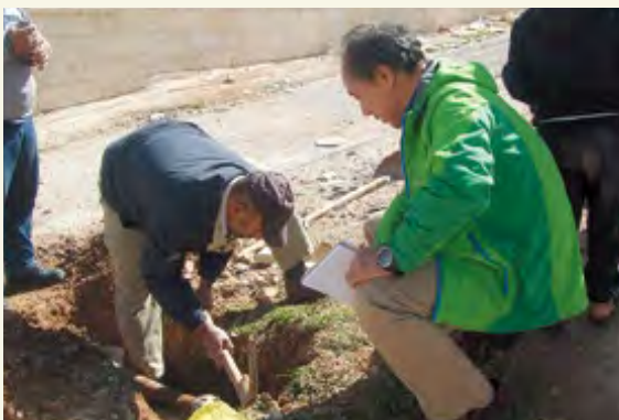
Yarmouk Water Company (YWC) officials check leakage from water pipes.
