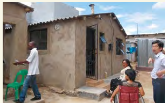
Houses being renovated with a ramp to be added for disabled people
