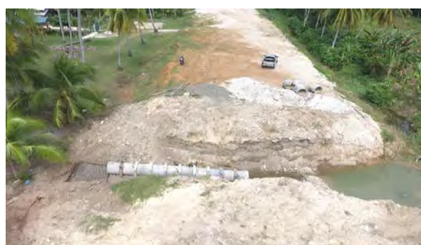
Photo shows the drainage pipe crossing at Sta. 0+120 of MC-3, which is the facility for drainage canal to cross the irrigation canal. Source: NIA-PMO
