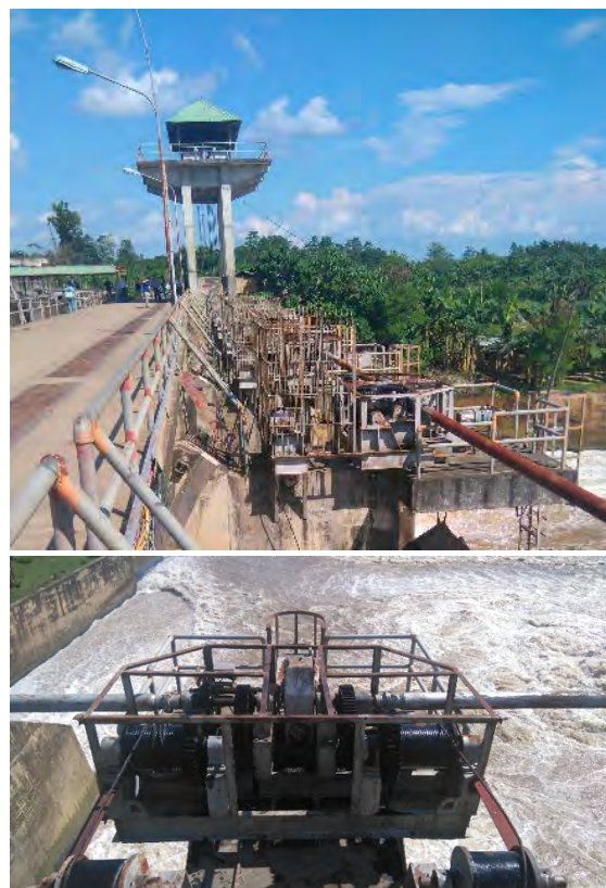
Above pictures show a gate lifting device at spillway. There is no shade to protect them from rain and sunshine, and metal parts of the device rust easily. Actually, in seven devices, the cable is already rusty and broken and the lifting devices are not working properly. The operation of these devices is at risk, hence the operation of the entire dam.
