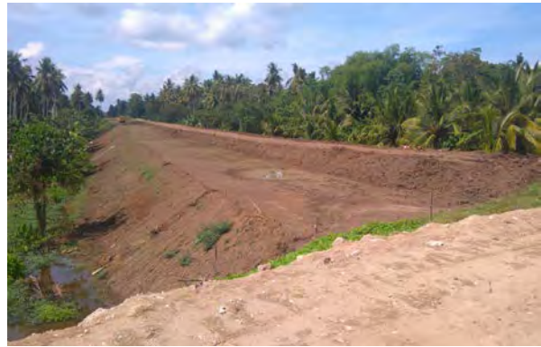
An example of dike constructed in MMIP II (MC-2 Main Canal), height goes up more than 5.0 m.
