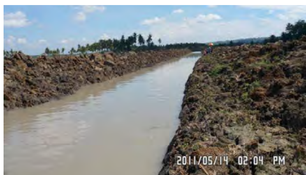
Photo shows the lateral drainage canal (LDC-PR-III) excavated in 2011 to improve the drainage capacity. Source: NIA-PMO
