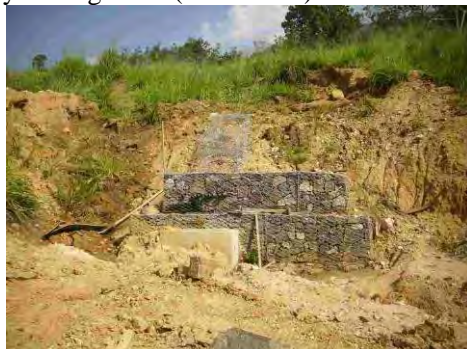
Small landslide behind the gabion wall caused by cutting work (Point No.1)
