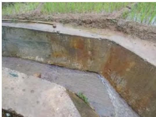
Photo 7: Erosion at the connecting point of base concrete and side wall. Repaired once, but eroded (Loc. 11)
