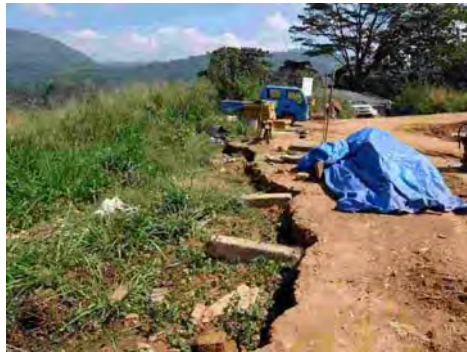
Cracks at the shoulder of the slope caused by cutting work (Point No.4)
