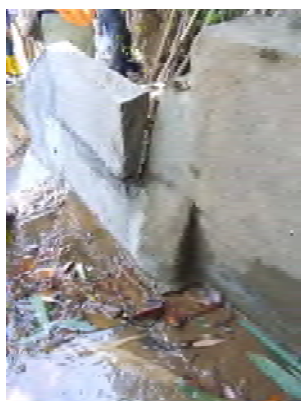
Photo 3: The ditch lower part of the pit has not been constructed properly. After the inspection, it has been corrected.(Loc. 3)
