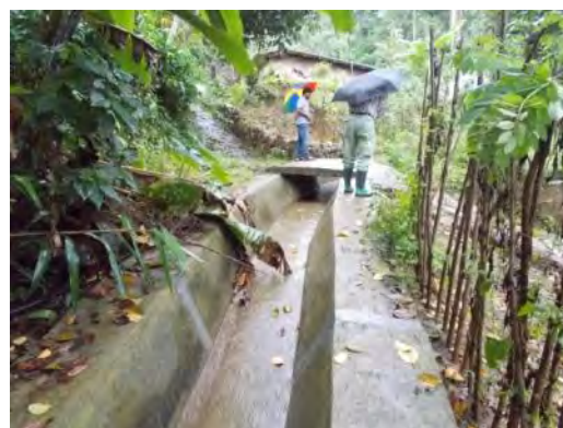
Photo 10: Crack along the expansion joint has been corrected. (Loc. 8)
