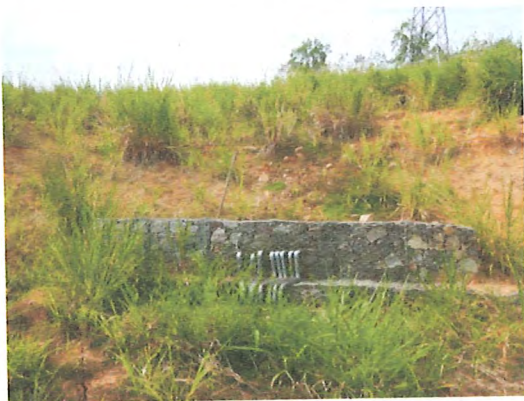
Photo 3: Small slip has been reshaped (D. P. 1)
