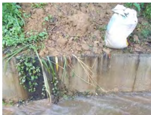
Photo 8: Eroded part was repaired once, but it is very difficult to find the exact place of erosion. (Loc. 12)
