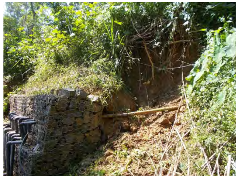
Photo 12: Collapse at the right side of gabion wall. (Horizontal drainage drilling No.10 was repaired)
