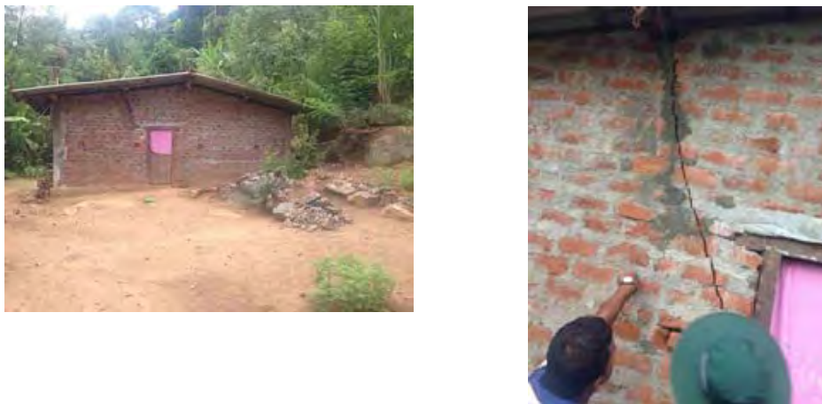
Photo 4.10 Cracks appeared on the wall of the house
