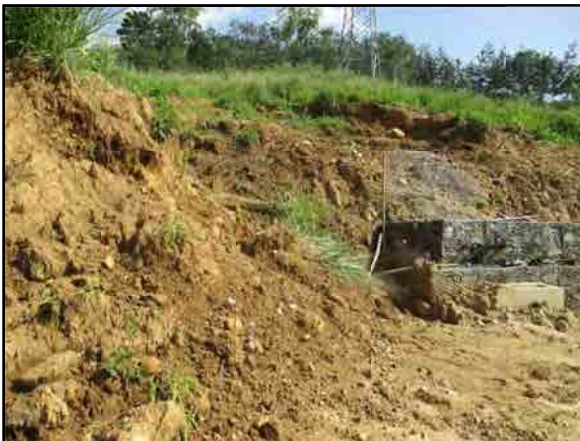
Earth collapse at location 1
