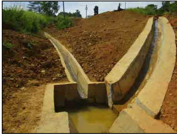
ype 2 catch pit constructed mid down the drain where types D and E drains join together
