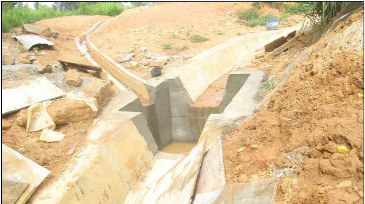
Type 3 catch pit constructed far down the drain where types B and E drains join together
