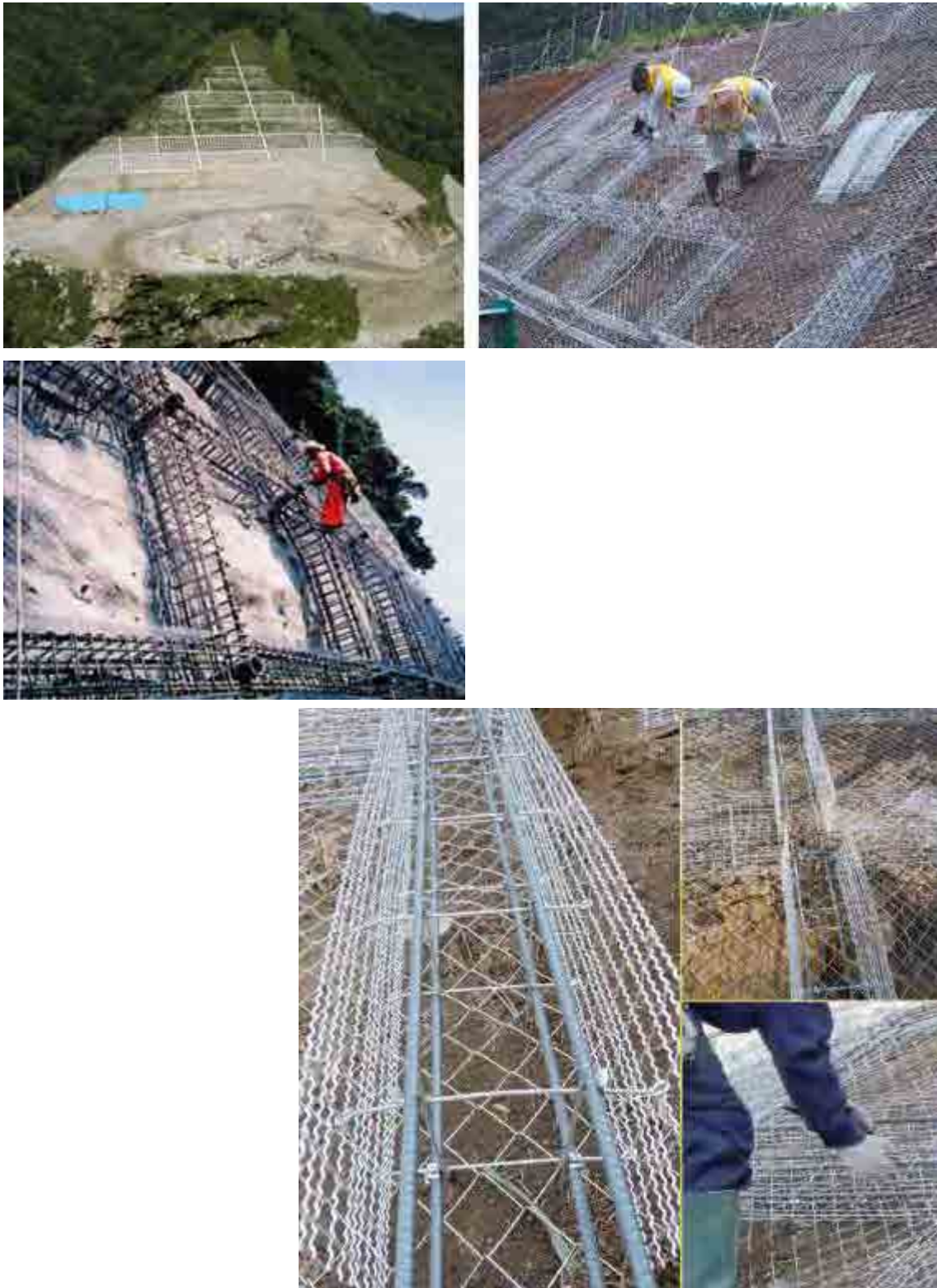
Photo 4 Example of grating crib works in Japan (Source: Web site of OKABE Co. Ltd; Top, Web site of Shiisaka Kensetsu; Middle, Web site of Free Frame Association; Bottom)
