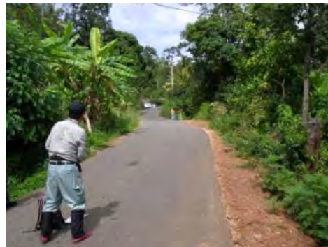
The gap of road surface formed due to landslide movement
