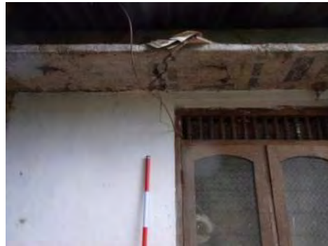
Crack caused by landslide on the residence wall
