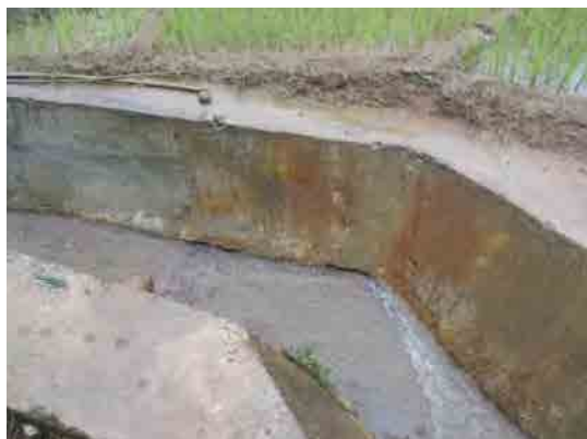
Photo 7: Erosion at the connecting point of base concrete and side wall. Repaired once, but eroded (Loc. 11)
