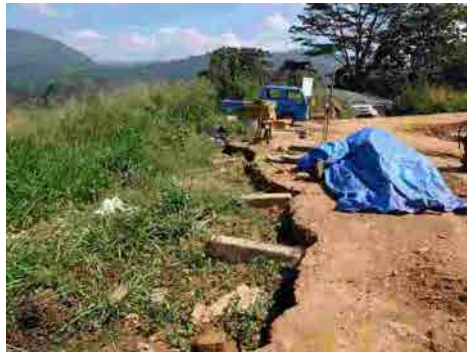
Cracks at the shoulder of the slope caused by cutting work (Point No.4)
