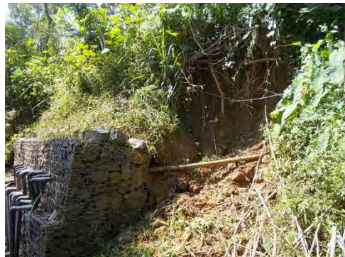
Photo 12: Collapse at the right side of gabion wall. (Horizontal drainage drilling No.10 was repaired)
