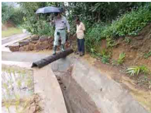
Photo 5: Crack on the ditch has been corrected. (Loc. 9)
