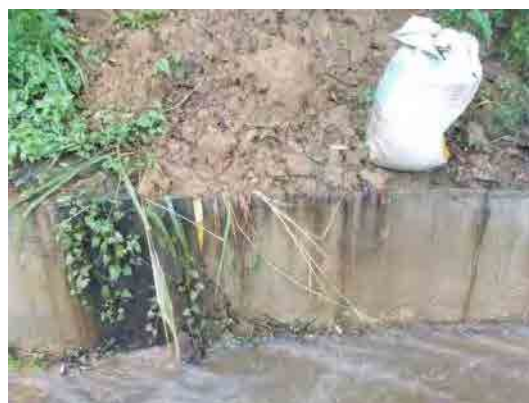
Photo 8: Eroded part was repaired once, but it is very difficult to find the exact place of erosion. (Loc. 12)
