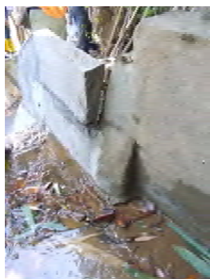
Photo 3: The ditch lower part of the pit has not been constructed properly. After the inspection, it has been corrected.(Loc. 3)
