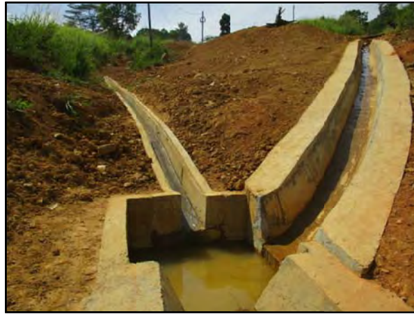
type 2 catch pit constructed mid down the drain where types D and E drains join together
