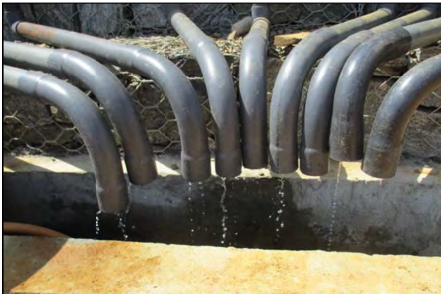
Water flowing down PVC pipes to catch pit at location 4
