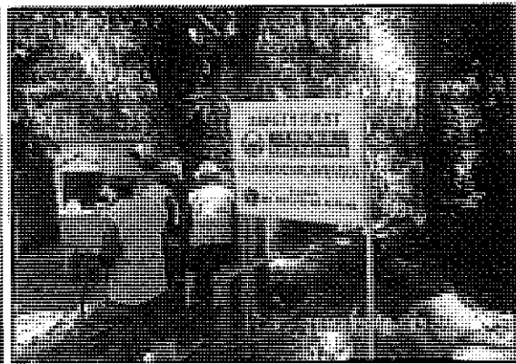
Fig 11: Safety Sign Board within the site
