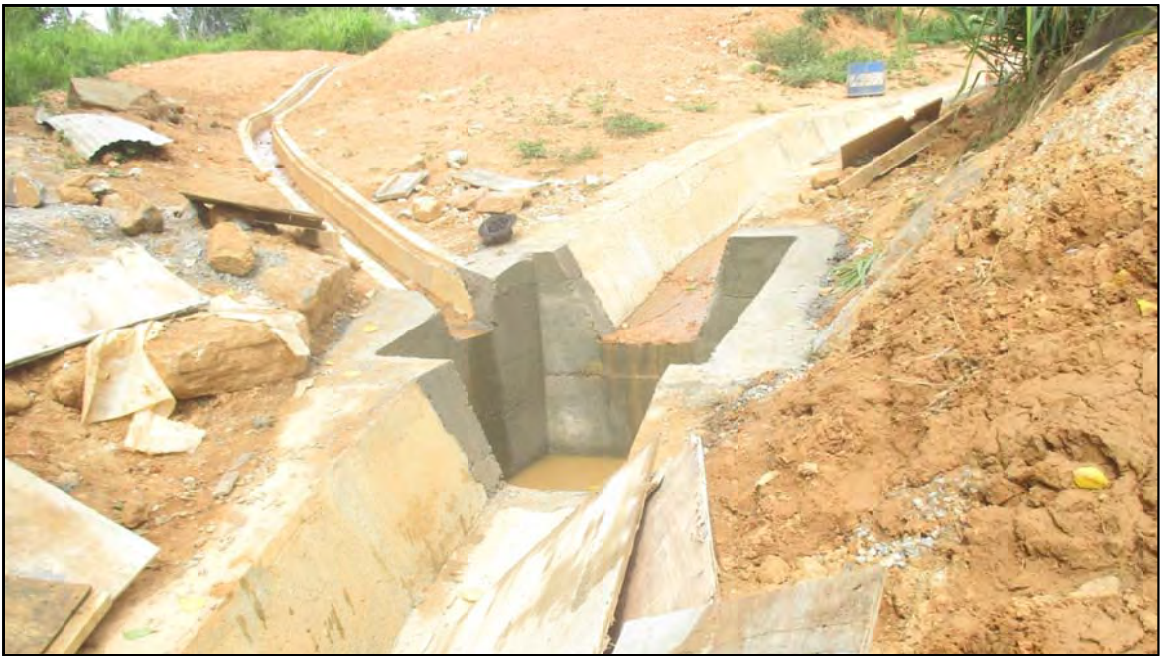
Type 3 catch pit constructed far down the drain where types B and E drains join together
