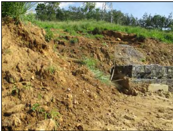
Earth collapse at location 1
