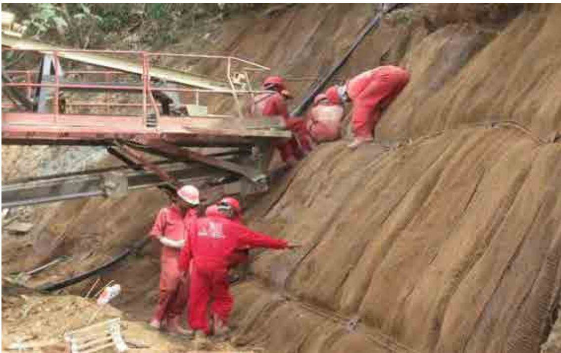
Photo 1 Example of grating crib work in Sri Lanka (Source: Web site of Soil Tech Ltd)
