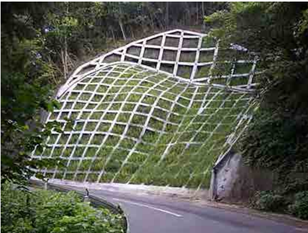
Photo 3 Example of grating crib works in Japan (Source: Web site of Higashiryokkakaihatsu Co; Upper, Web site of Aura C. E; Lower)
