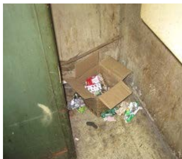
Photo 2.4-118 Garbage littering electrical plant room
