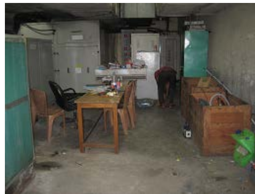
Photo2.4-128 Contractor work location (Air conditioning plant room)
