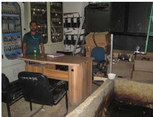
Photo2.4-127 Contractor work location (Air conditioning plant room)
