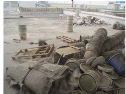
Photo 2.4-74 Scattered Rubbish on the Roof of the Terminal Building
