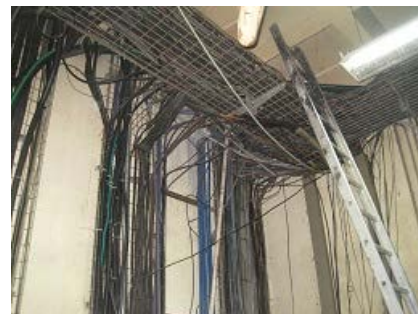
Photo 2.4-117 Wiring in electrical plant room
