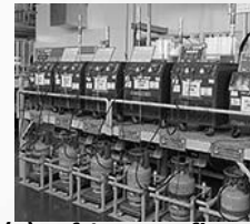
(F) Refrigerant fluorocarbon gas collection
