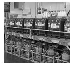
(F)Refrigerant fluorocarbon gas collection
