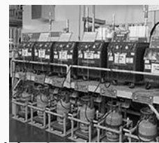
(F)Refrigerant fluorocarbon gas collection
