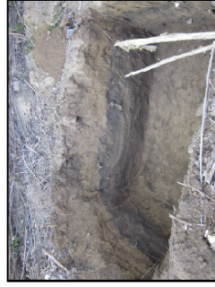
Temporary Sedimentation Pit
