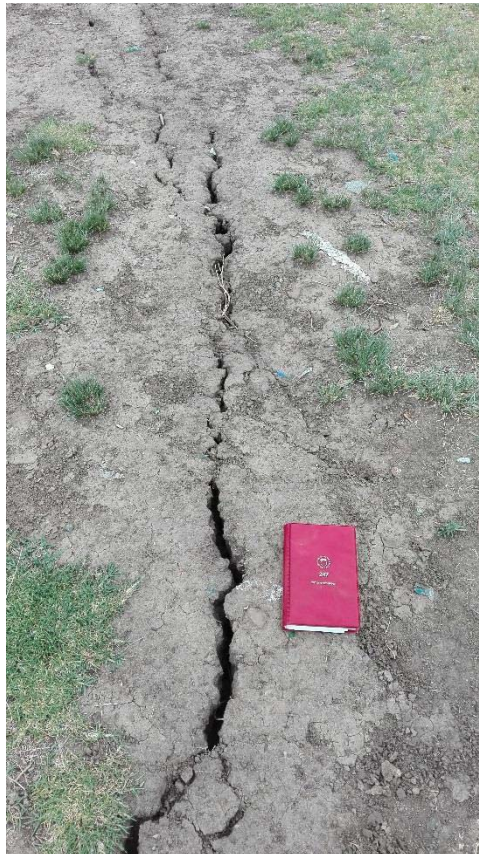
Plate 4 : Very widely open desiccation cracks at ground level within the active clayey subsoils.
