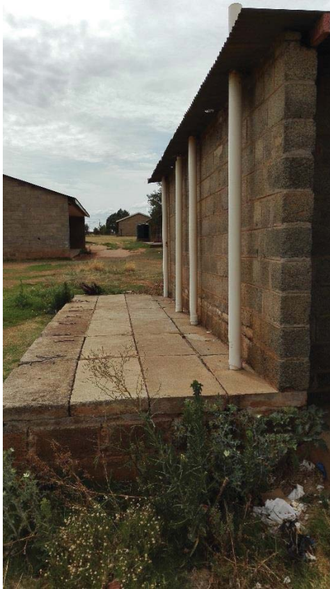
Plate 3 : Example of existing permanent pit latrines on site with single storey school structures located in background.
