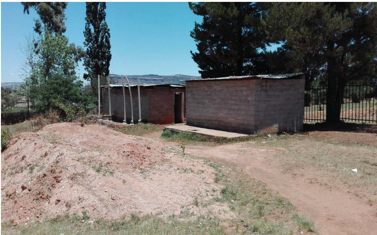
Plate 4 : Existing Pit latrine ablution facilities located at south western corner of the site.
