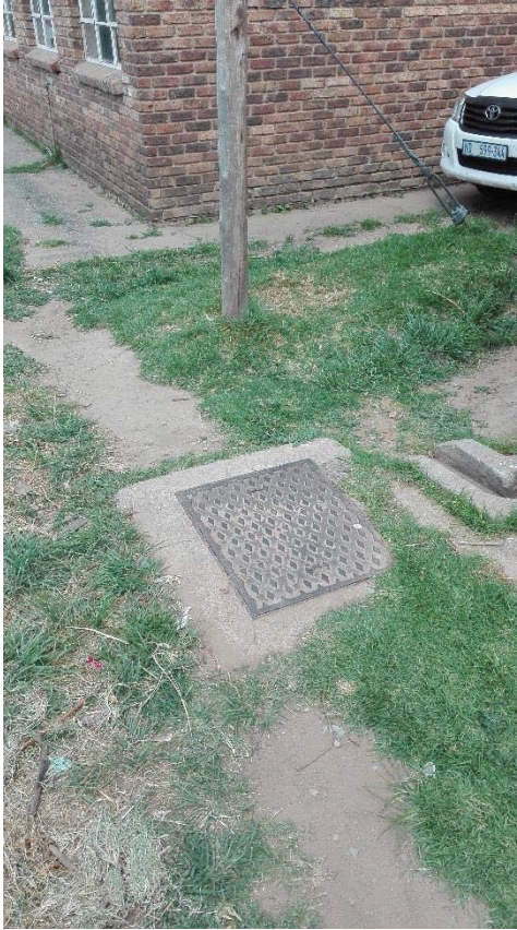
Plate 3 : Example of manhole for possible sewerage / storm water disposal system existing on site.
