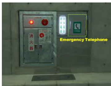
Emergency Telephone on wall
