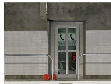
Emergency Telephone Box
