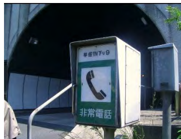
Emergency Telephone at Entrance
