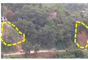
(5) Slope Failure at Sanga Pass (27 August 2015)
