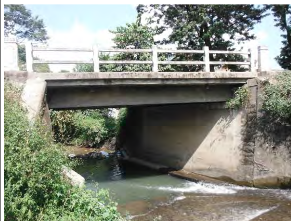
Photo-10: Existing bridge at Jagati city (Over 40 years after construction, degradation progresses, breakage is seen)
