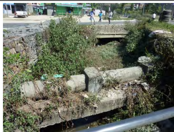
Photo-19: Existing bridge and sewer bridge at Banepa city (Over 40 years after construction, degradation progresses, breakage is seen)
