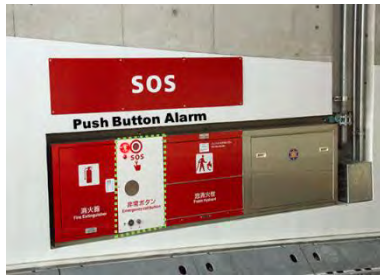
Push Button Alarm with Fire Extinguisher & Fire Hydrant
