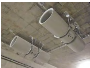
Smoke Removal System (Jet Fan)
