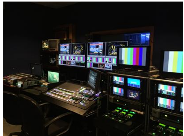
Control facility (MTV)
