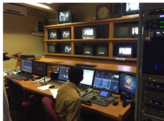
Master control facility (Voice of Asia)
