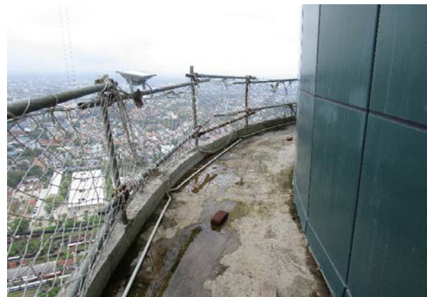
Micro platform where parabolic antenna will be installed
