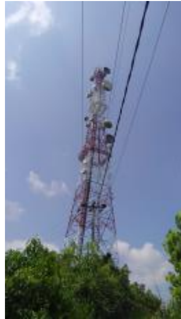
Antenna Tower in Elpitiya
