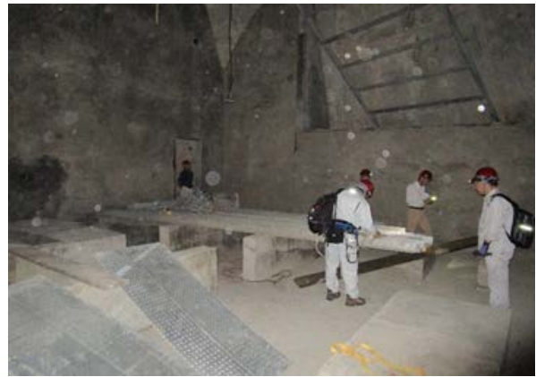
Confirmation of route for laying cables at water storage floor in Tower House
