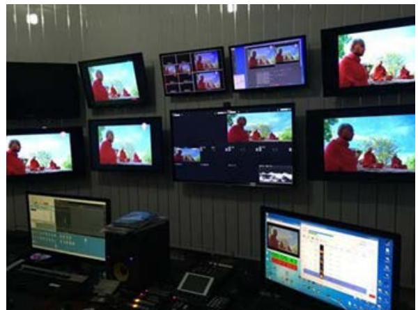
Master control facility (Shradda TV)
