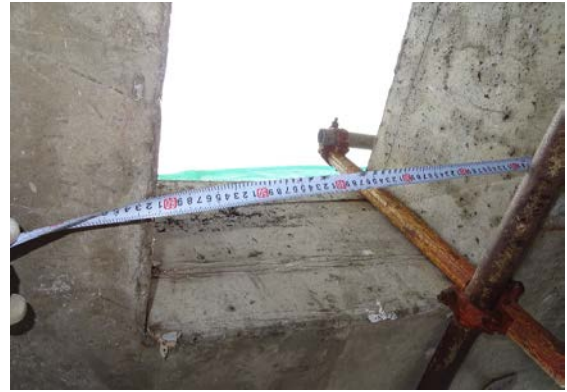
Measurement of size of hole for carrying up antenna panels from Tower House to antenna mast
