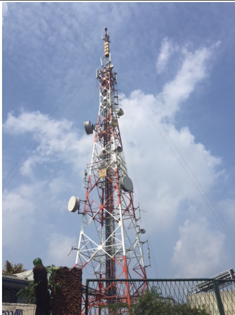
Antenna tower in Kurunegala
