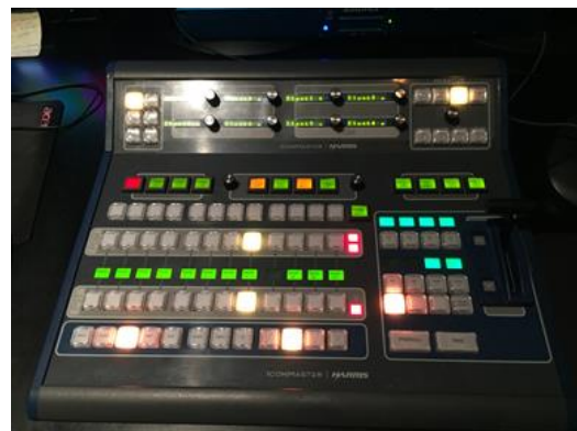
Master control facility (CSN)
