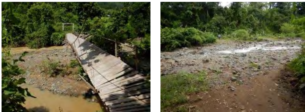
Figure 3-1-4 Existing suspension bridge at Road A (Damaged) and river crossing point for agricultural machine at Road B
