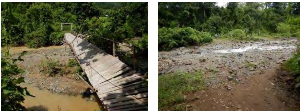
Figure 3-1-4 Existing suspension bridge at Road A (Damaged) and river crossing point for agricultural machine at Road B
