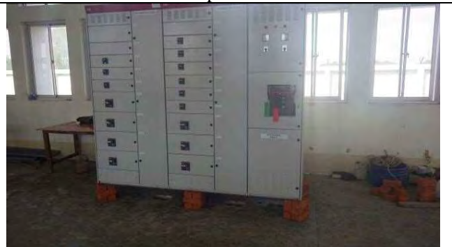
Incoming panel, 28 May 2017
