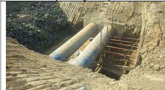
Flowmeter chamber, 21 Feb. 2017
