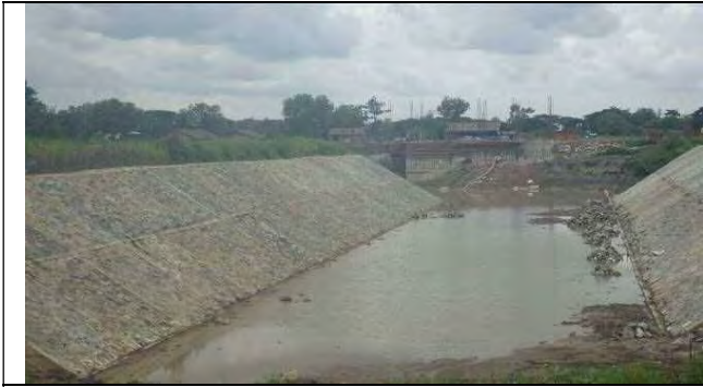
Grit chamber, 04 Sep. 2015
