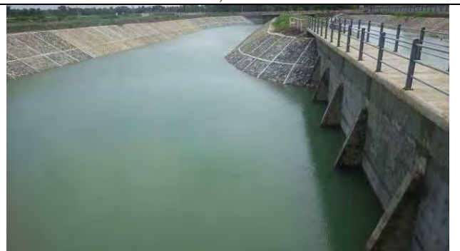
Grit chamber, 09 June 2016
