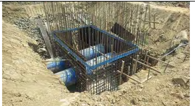
Flowmeter chamber, 09 March 2017
