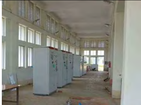
Control panel, 27 Oct. 2017
