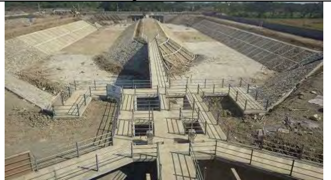
Grit chamber, 29 Feb. 2015
