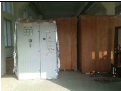
Incoming panel/ Control panel, 29 Sep. 2017
