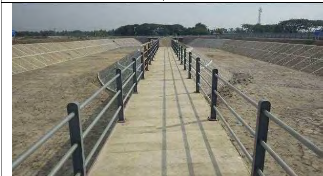
Grit chamber, 29 March 2016
