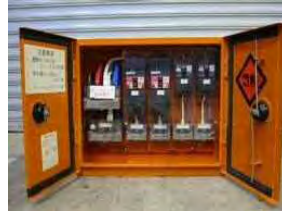
Switch board Recommended to use on site
