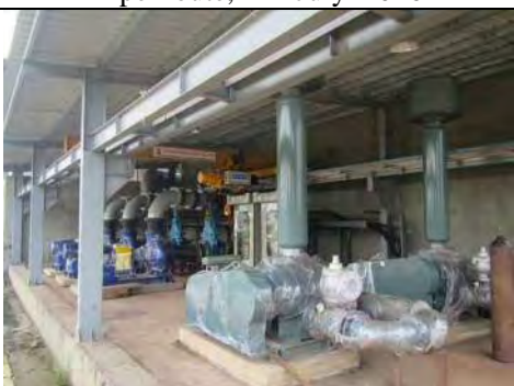
Back wash pump and blower, 28 Sep. 2016
