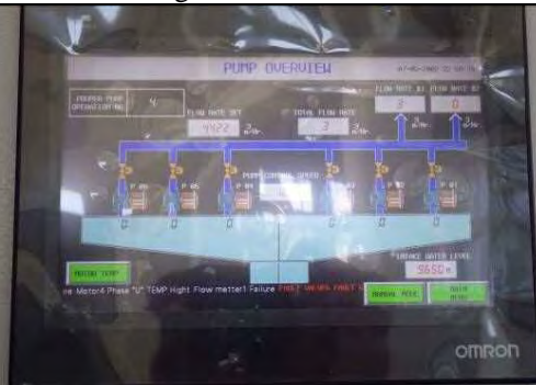
Check of control program, 11 Jan. 2018
