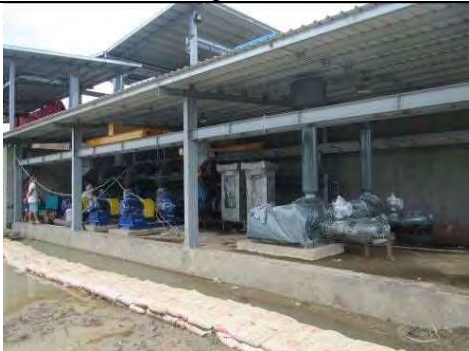
Back wash pump and blower, 07 July 2016
