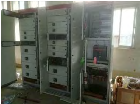
Control panel, 21 Jan. 2017
