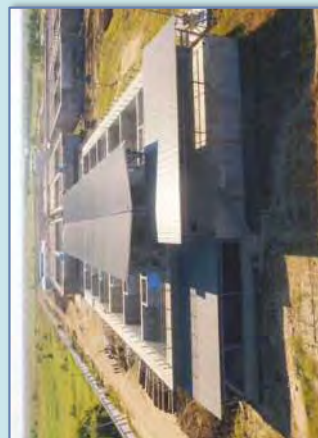
Rapid Sand Filter Super Structure
