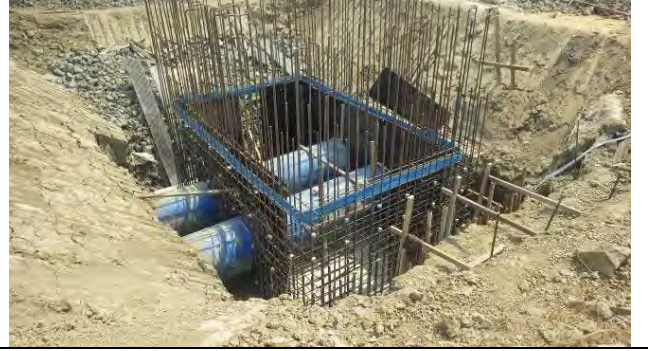
Flowmeter chamber, 09 March 2017
