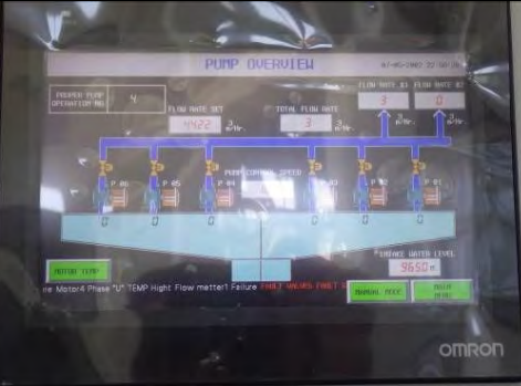
Check of control program, 11 Jan. 2018
