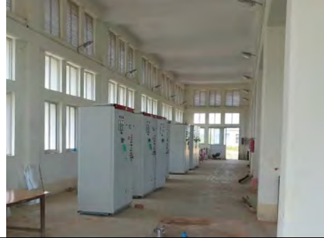
Control panel, 27 Oct. 2017
