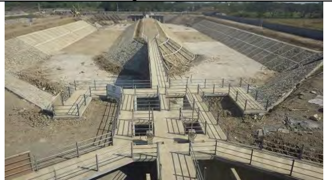
Grit chamber, 29 Feb. 2015
