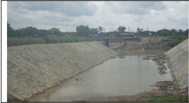
Grit chamber, 04 Sep. 2015
