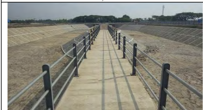
Grit chamber, 29 March 2016
