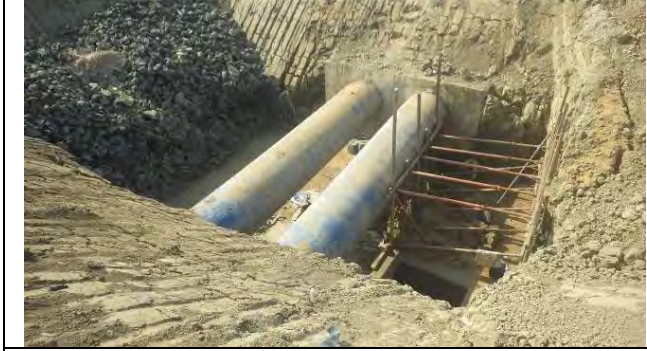
Flowmeter chamber, 21 Feb. 2017
