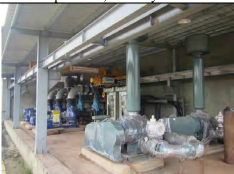
Back wash pump and blower, 28 Sep. 2016
