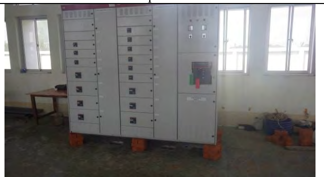
Incoming panel, 28 May 2017
