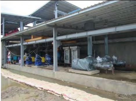
Back wash pump and blower, 07 July 2016
