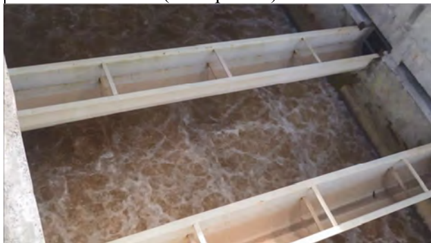
Air Backwash by Improved Strainer (22 Sep 2017)
