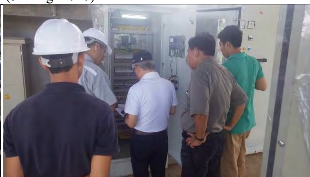
Test Operation of Control Panel (13 Oct. 2016)
