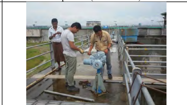
Malfunction of Discharge Valve on Filter Tank (28 Jul 2017)
