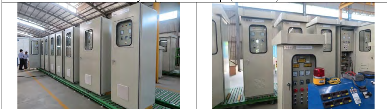
Factory Inspection: Electrical Panels (22 November 2015)
