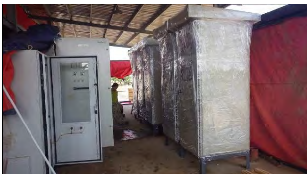
Control Panel (02 June 2016)
