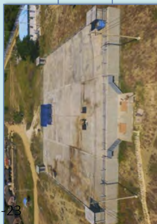
Clear Water Reservoir
