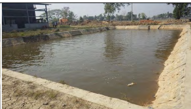
Water Discharged from Drainage Tank to Lagoon (13 Mar 2018)
