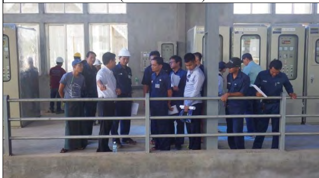
Training on Lift Pump Maintenance & Inspection (09 Sep 2016)
