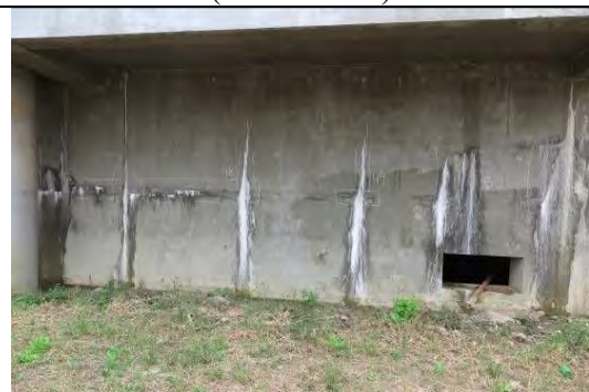
Leakage Condition of Sedimentation Tank (07 Dec 2016)
