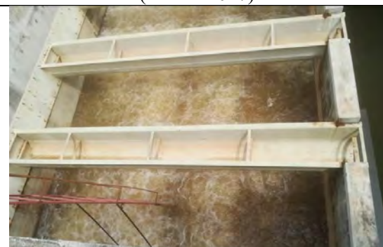
Air Backwash by Improved Strainer (17 Oct 2017)
