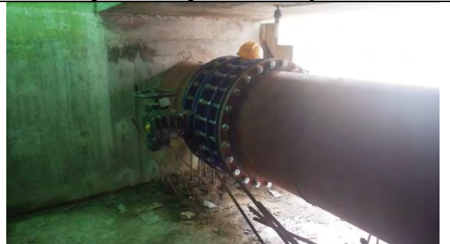
Inlet valve, 13 Oct. 2016
