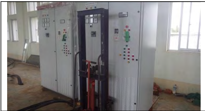
Incoming panel, 07 Sep. 2017
