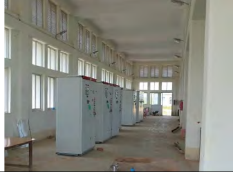
Control panel, 27 Oct. 2017
