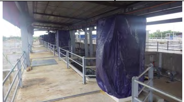
Control panel, 21 July 2016
