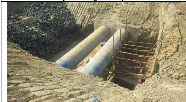
Flowmeter chamber, 21 Feb. 2017
