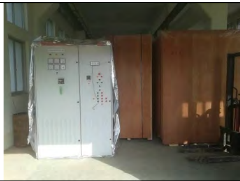
Incoming panel/ Control panel, 29 Sep. 2017
