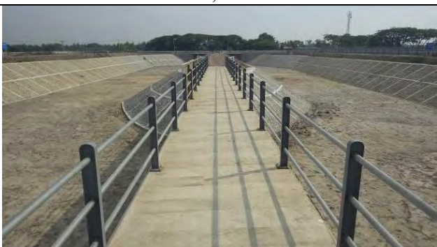
Grit chamber, 29 March 2016
