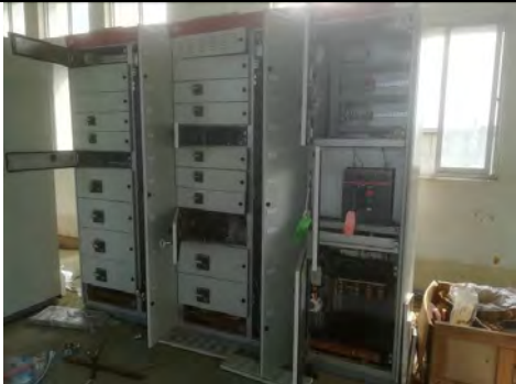
Control panel, 21 Jan. 2017
