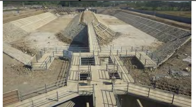
Grit chamber, 29 Feb. 2015
