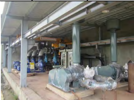
Back wash pump and blower, 28 Sep. 2016
