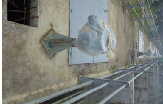
Drain valve, 21 July 2016
