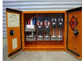
Switch board Recommended to use on site
