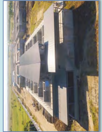
Rapid Sand Filter Super Structure
