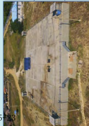
Clear Water Reservoir
