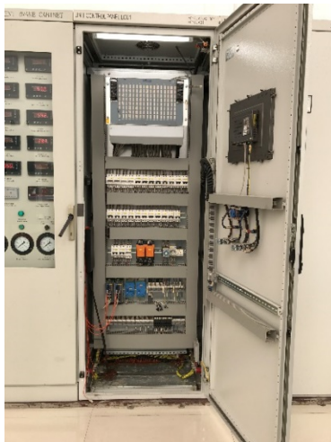
UNIT CONTROL PANEL
