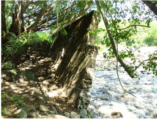
Flood wall (destroyed)
