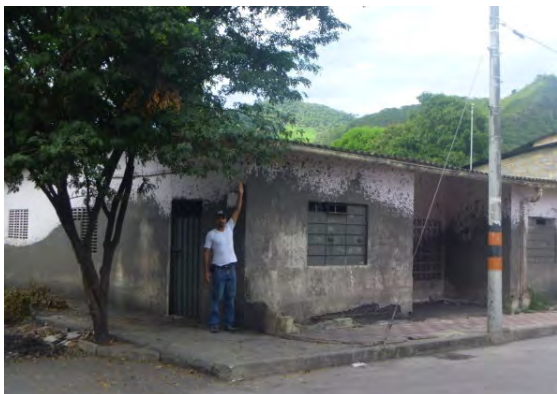
Image No. 2.29. Effects of the hydrogeomorphological event of April 18, 2011: Flood footprint in housing (up to 2.25 m).
